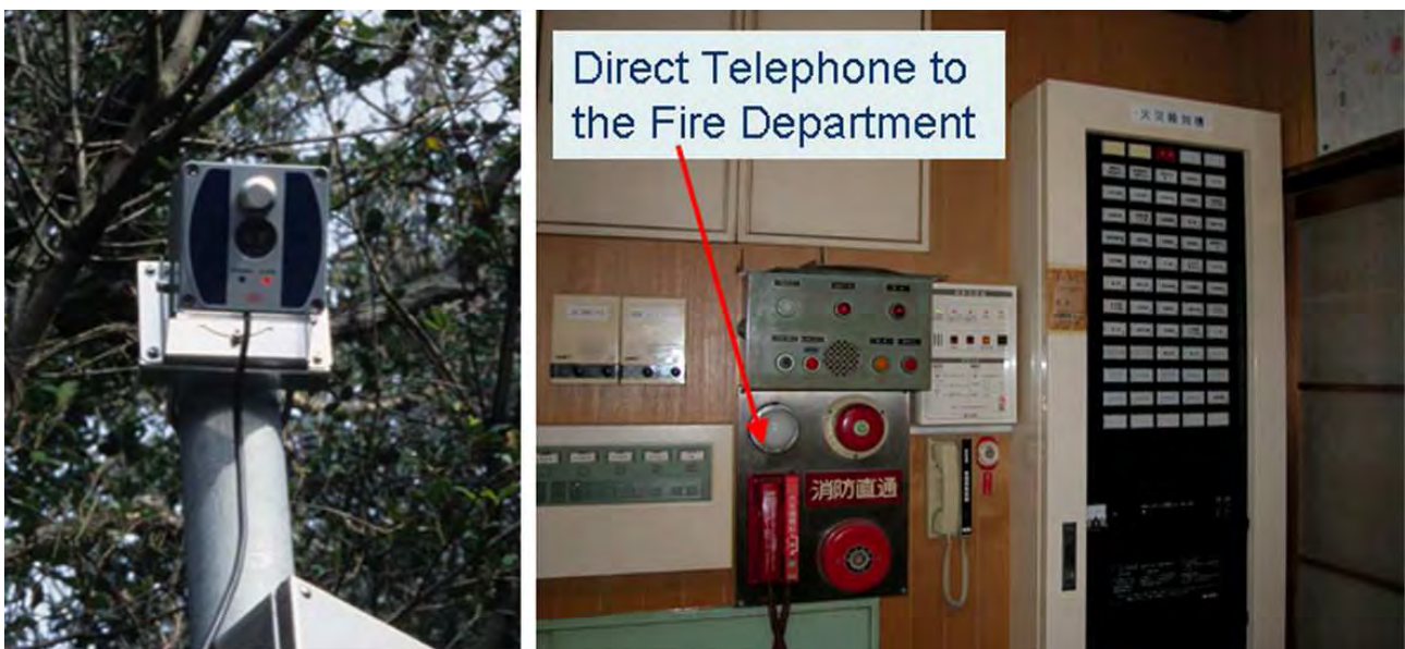
Fig. 2. Flame Detector (left) and Direct telephone lines to the fire department (right)
