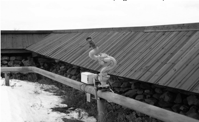
Fig. 5. Fire pipeline. Fire monitor. (A. Ljubimtsev)
