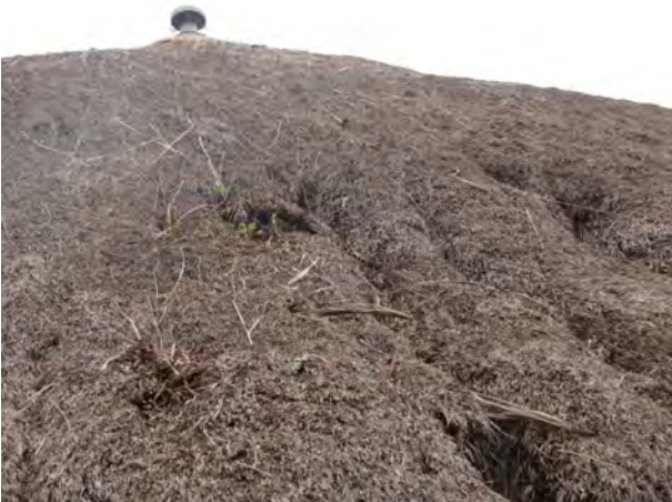
Fig. 5 Damages to grass roof
