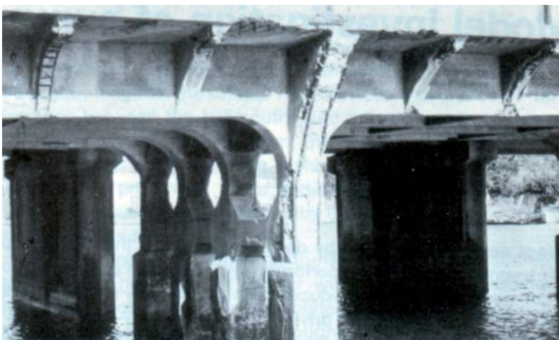
Concrete bridge in serious need of maintenance.
