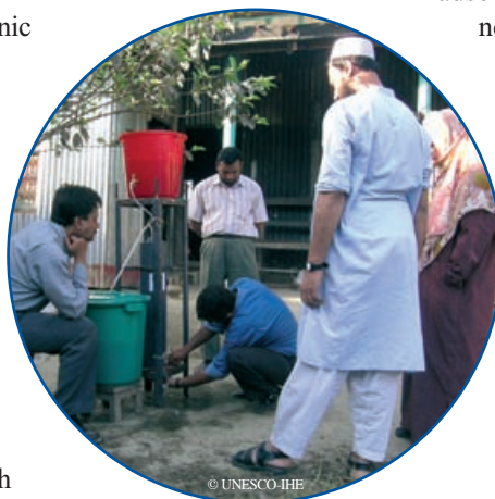
Installation of one of the family filters in the garden of the 10-member Gafur family, in Dhunshi
