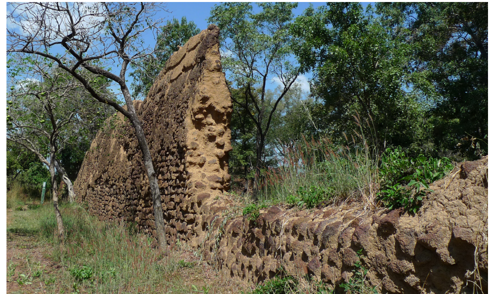
Tear on west wall © David Gandreau, CRAterre
