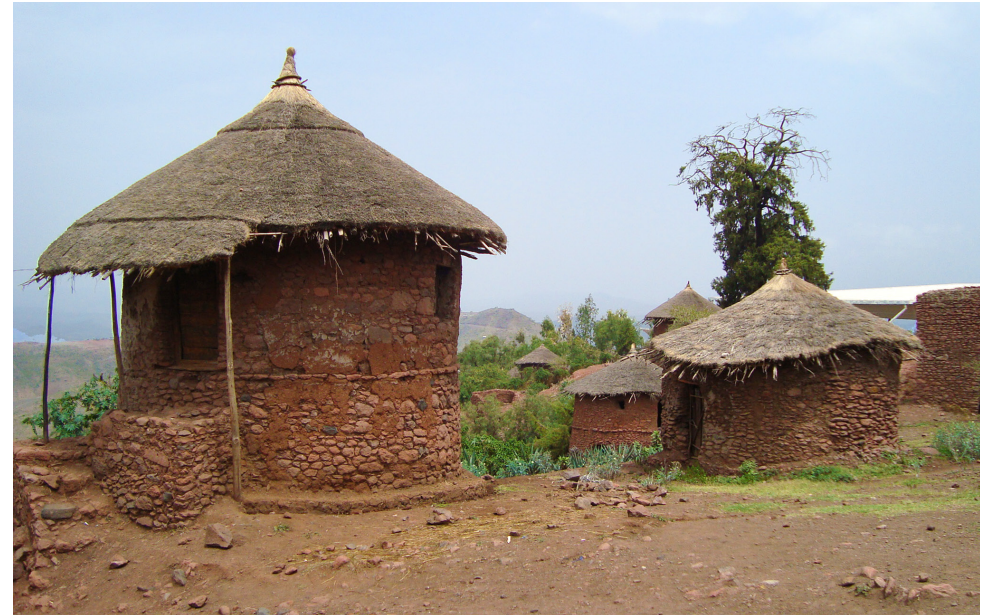
A Tuluk is a round, two-level house, built of stone and earth walls. The example above shows that the earthen plaster covering the wall is almost gone © Ishanlosen Odiaua
