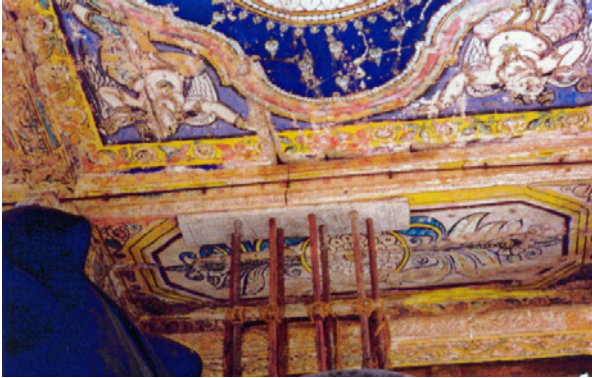
View of Cracks in the Nandi Mandapa ceiling before restoration
