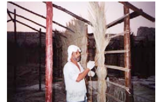
F11- P31- CONSERVATION OF THE TRADITIONAL BARASTAJ ON THE UPPER LEVEL OF THE MAIN FORTRESS ("BAHRAIN FORT") (DECEMBER 2003)
