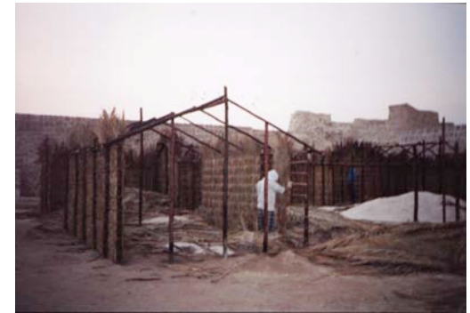
F11- P29- CONSERVATION OF THE TRADITIONAL BARASTAJ ON THE UPPER LEVEL OF THE MAIN FORTRESS ("BAHRAIN FORT") (DECEMBER 2003)
