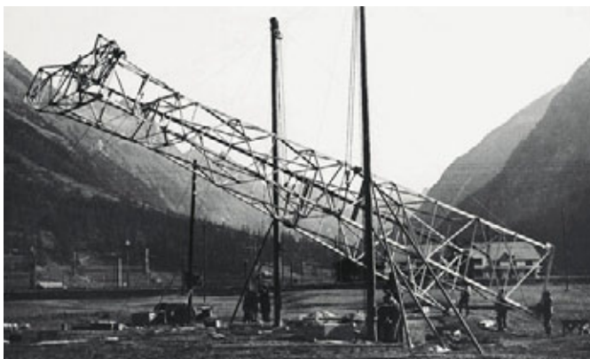
The Rhätische Werke Thusis built a power line over the Albula Pass in 1921. This created a link with the south; with the Brusio power stations. The photograph shows the erection of the iron masts in the Engadin. Rätia Energie AG, Poschiavo
