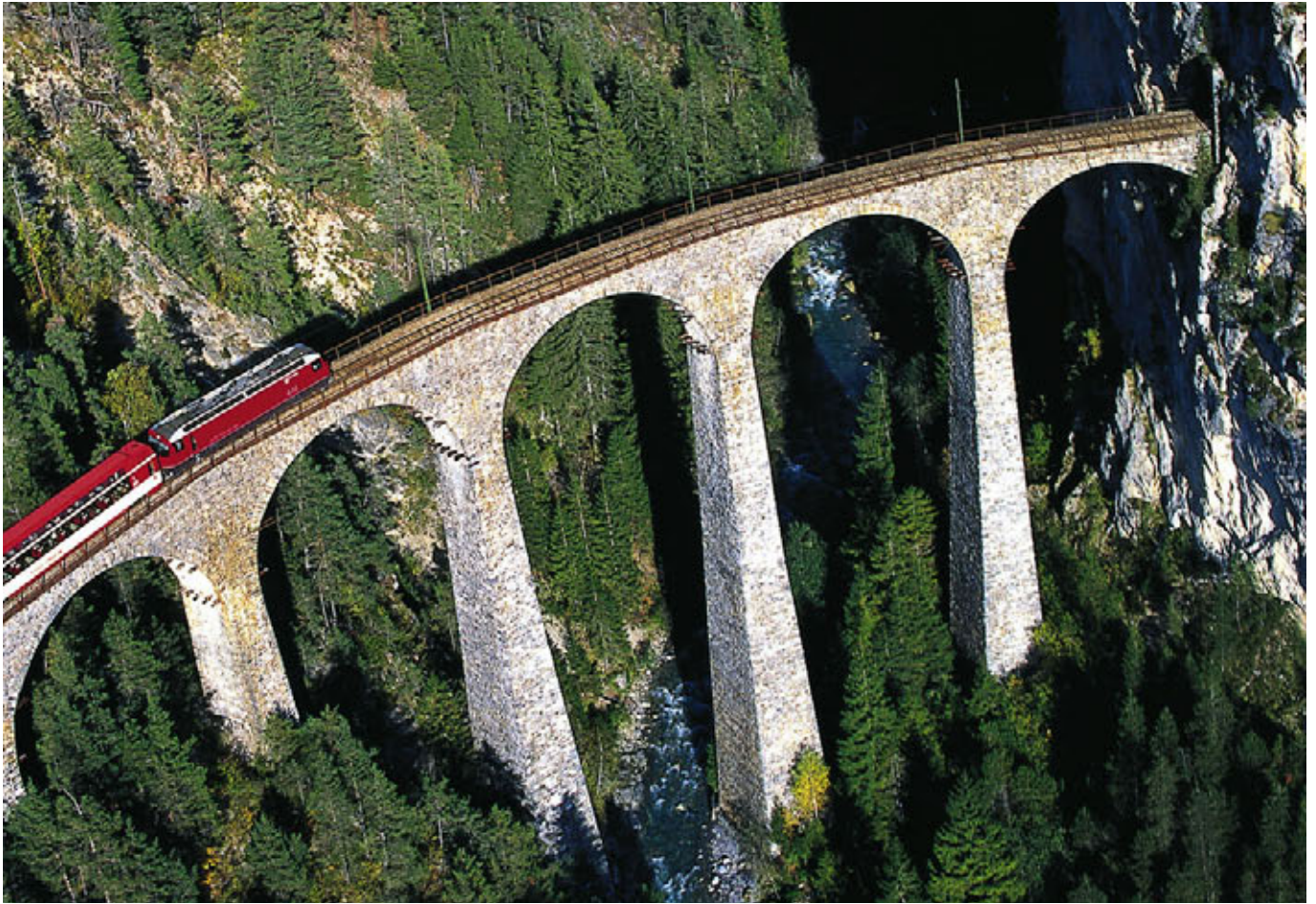
Albula line > Landwasser Viaduct. The Landwasser Valley is crossed at the narrowest point with a radius of only 100 m. P. Donatsch
