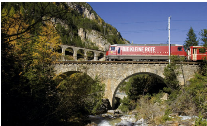
Albula line > In the foreground the 11 m high and 59 m long Albula Viaduct I. In the background left, the Rognux inclined viaduct. A. Badrutt
