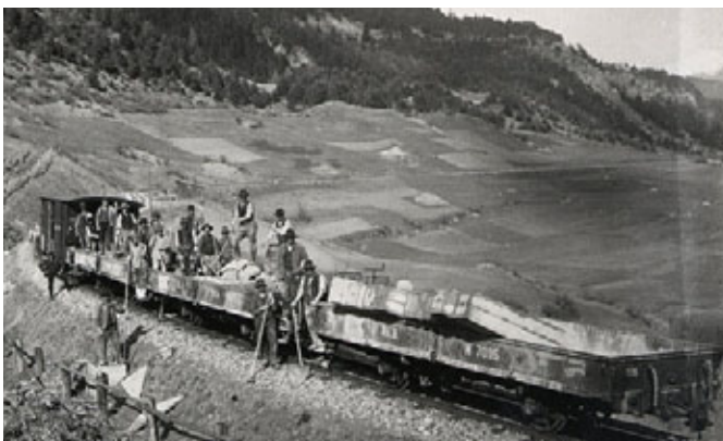
Electrification of the Albula line > Catenary works-train between Surava and Tiefencastel: photograph about 1918. Collection G. Brüniger
