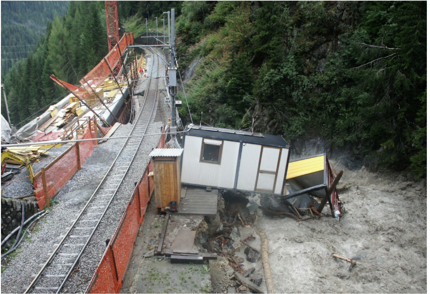
Val Tasna Viaduct > In August 2005, the old bridge collapsed in a great storm before the new parallel structure was finished. The new bridge was not damaged by the storm. Rhaetian Railway
