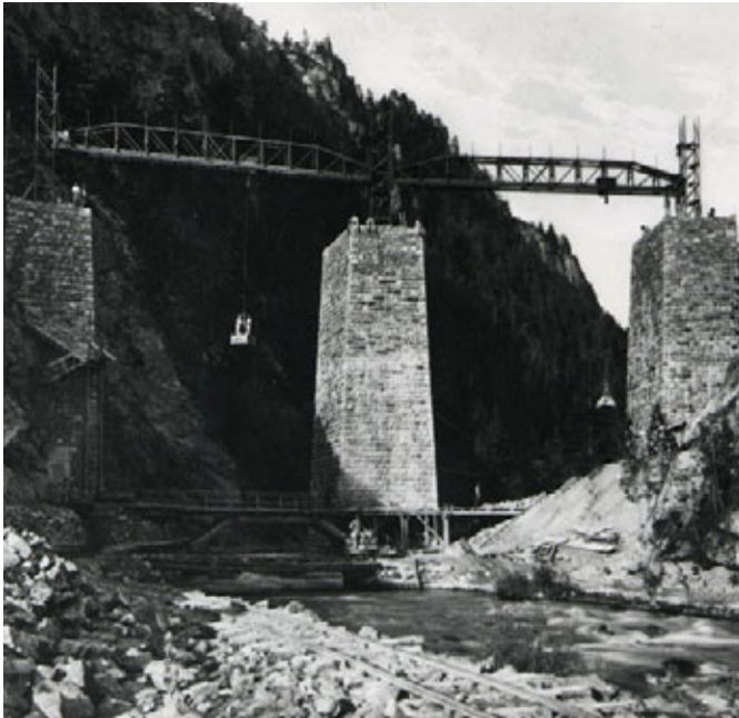
Albula line > Crane bridges were used for the construction of the Landwasser Viaduct. Photograph 1901. Rhaetian Railway
