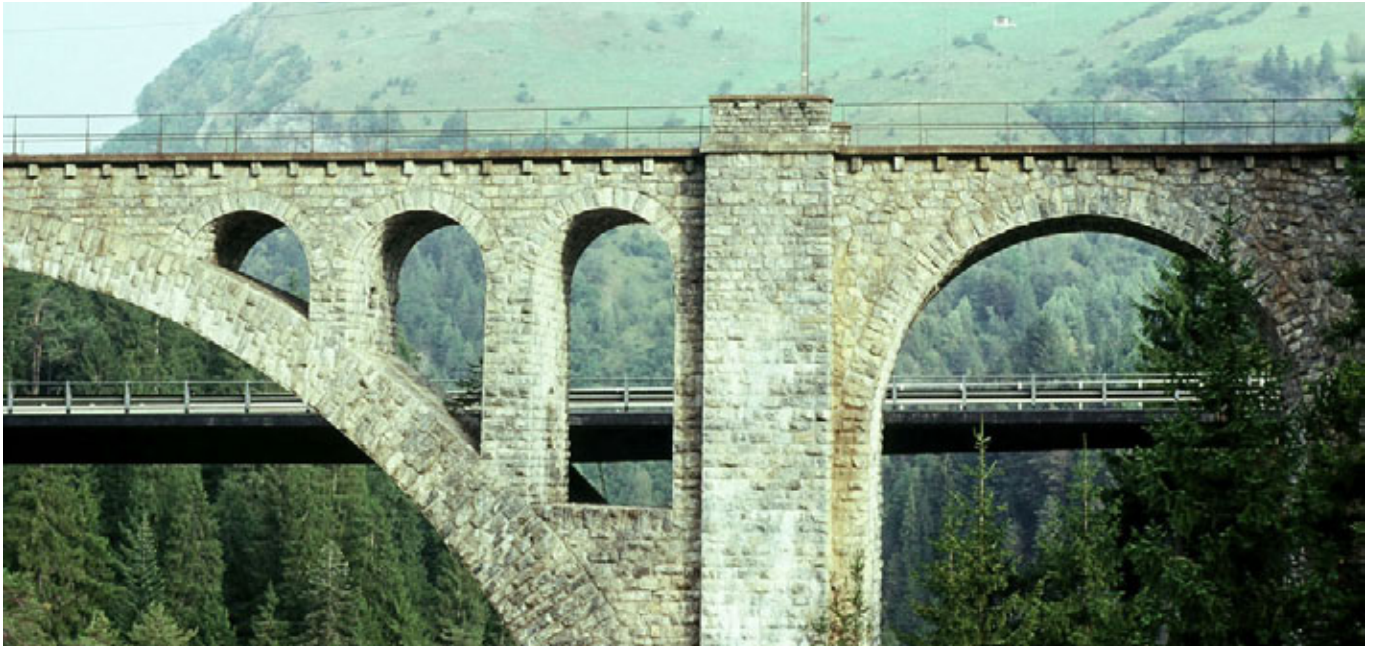
Albula line > A non-standard parapet was used for the Solis Viaduct that looks particularly delicate when viewed from the side. J. Conzett
