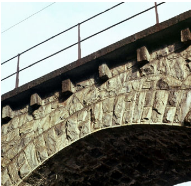
Solis Viaduct > Detail of the crown of the wall and the parapet. J. Conzett
