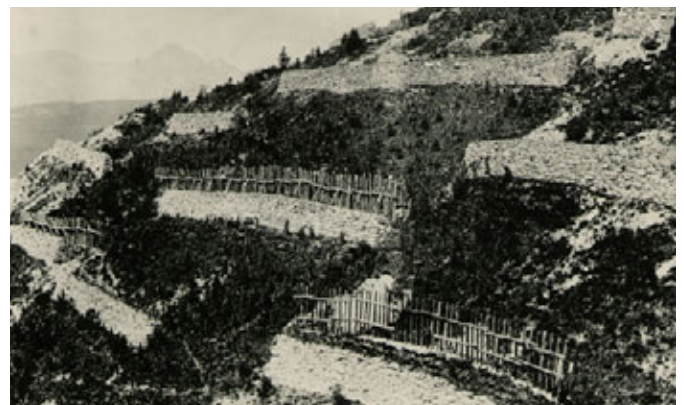
Albula line > Walls with snow catchers, Muot avalanche protection baffle. Rhaetian Railway
