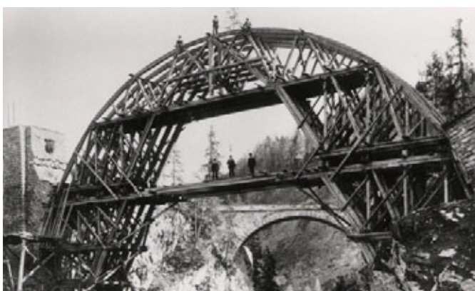
Albula line > Framework for the construction of the Solis Viaduct, erected by Richard Coray. Photograph 1901. Rhaetian Railway
