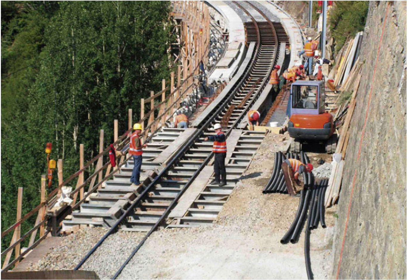
Rhaetian Railway > Laying the concrete ballast trough on the Val Lumpegna Viaduct in the Surselva, 2005. Rhaetian Railway
