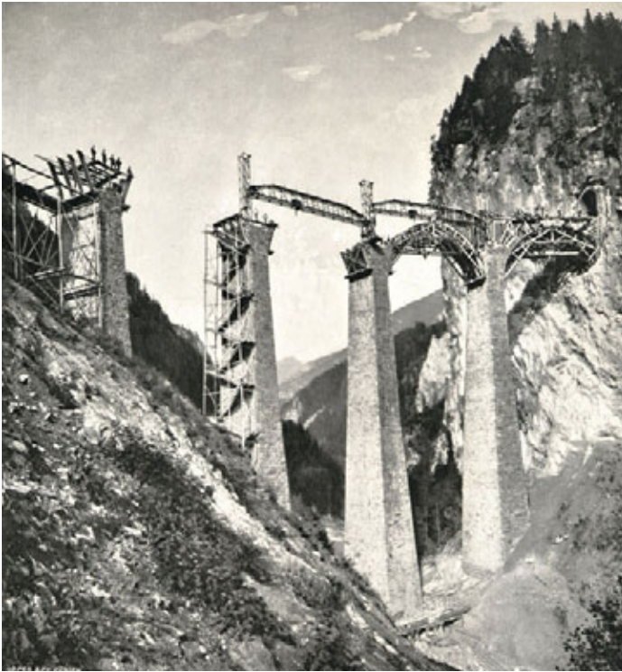
Landwasser Viaduct > The iron towers supporting the bridge cranes were built into the piers. This made it possible to do without construction frameworks in an area liable to flooding. Rhaetian Railway
