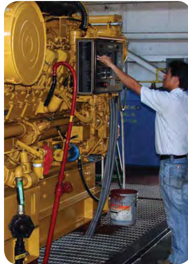
Caterpillar electric generator
