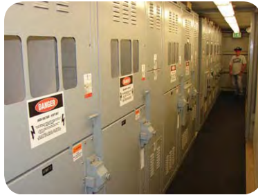
Electrical switch gear
