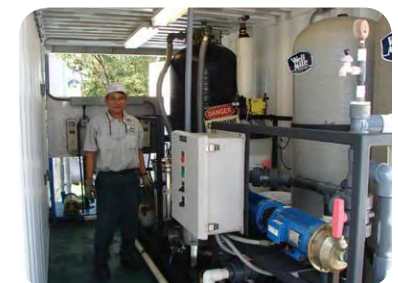
Water treatment facility
