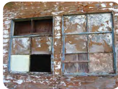
Peeling lead-based paint
