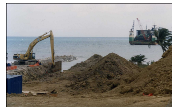
Pipe laying work in progress, Guayaguayare Bay, southeast coast of Trinidad (July 2003)
