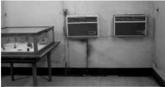
Figure 16. Typical small museum and the ubiquitous modern air conditioners. These often cause as much harm to artefacts as comfort to visitors and staff. They often cause high RH where it never existed before, and a source of water drips (condensation) where it never existed before.
