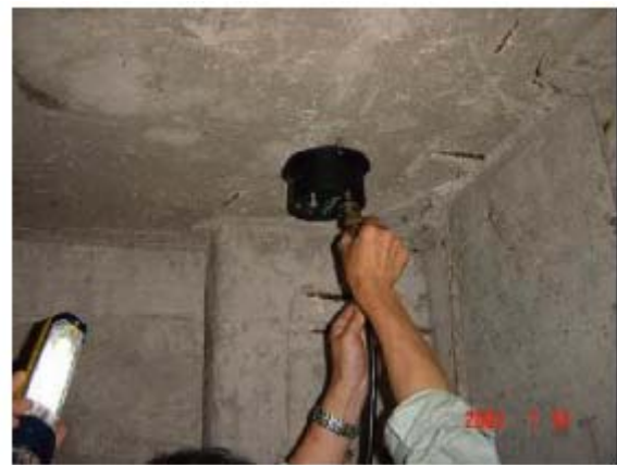
Figure 11. Seismic instrumentation of a building
