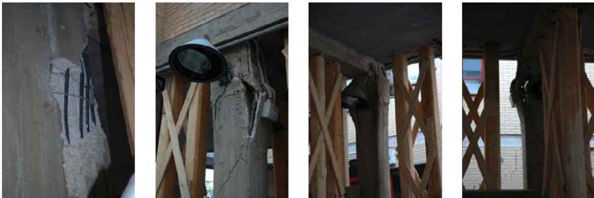
Figure 9. L'Aquila (April 2009): pillars in the San Salvatore Hospital, heavily damaged due to very inadequate steel reinforcement and poor concrete quality (no inert materials are visible in the pillar upper part)
