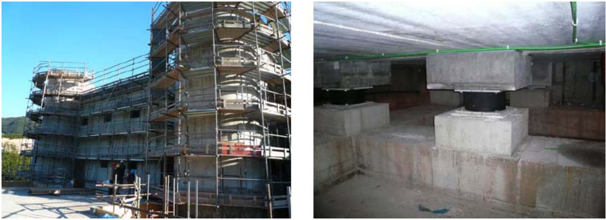
Figure 17. The new school of Marzabotto (Bologna), in seismic zone 3, under construction on HDRBs and SDs. Its safety will be certified by A. Martelli
