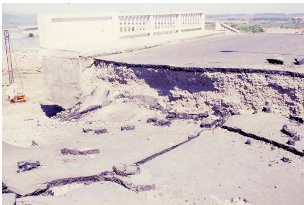
Figure A1. Settlement of embankment at the entrance of the Llo-lleo-Santo Domingo Bridge.
