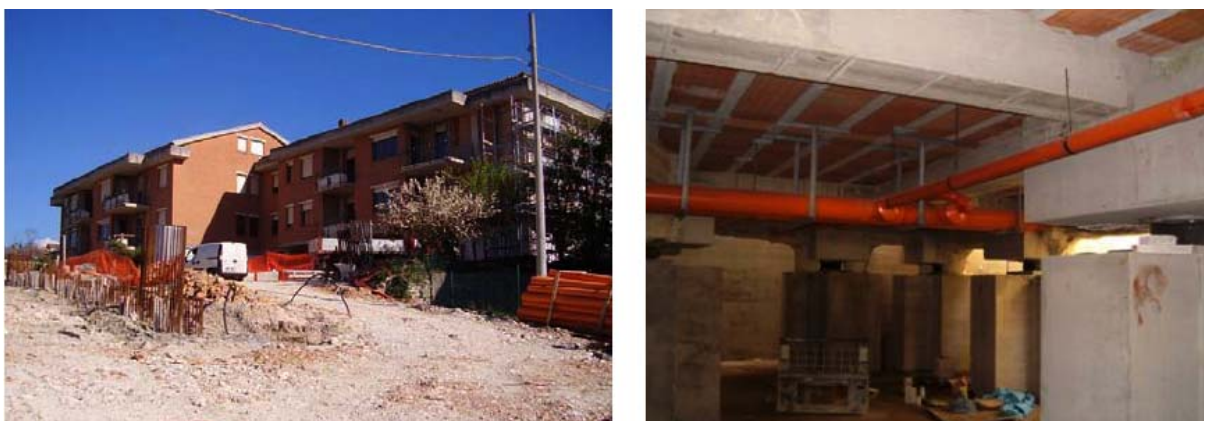
Figure 22. Three storey r.c. private house in Fabriano (Ancona), in seismic zone 2, damaged by the 1997-98 Marche and Umbria earthquake, first EU application of SI in a sub-foundation, the retrofit of which was completed with 56 HDRBs of 3 sizes in 2006, with safety certification of A. Martelli.
