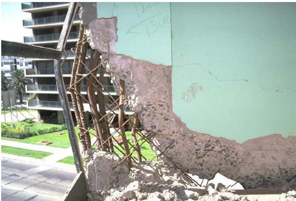
Figure A4. Acapulco Building in Viña del Mar. Detail of Damage in main Shear walls. Note the plain reinforcement bars.
