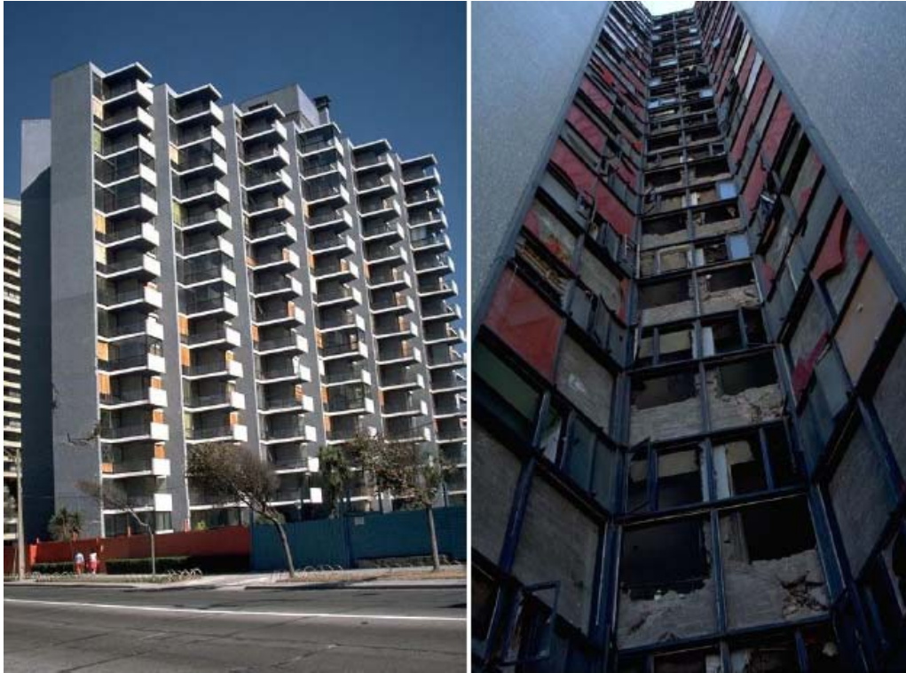
Figure A3. Acapulco Building in Viña del Mar. General View and Detail of Damage in Coupling beams. Building was erected in the mid 1960s and had already suffered some damage with a smaller earthquake in 1971.
