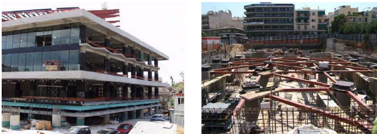
Figure 31. Recent Greek applications: the Onassis Centre at Athens , with the Acropolis Museum , isolated by 94 German SIP devices in 2006 (left), and Onassis House of Letters and Fine Arts , during its construction, again with German SIP devices, in 2007 (right).
