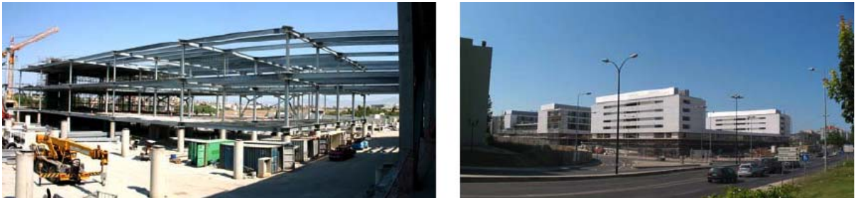
Figure 32. The Shakolas Park Commercial Centre at Nicosia (Cyprus), designed by the Italian GLIS and ASSISi member G.C. Giuliani and his son, formed by 2 buildings with mixed r.c. and steel structure, with 164 Italian HDRBs at top of the basement columns (left), and La Luz new hospital at Lisbon (Portugal), which was baseisolated, together with a residence for old people, by means of 315 Italian HDRBs in 2006 (right)
