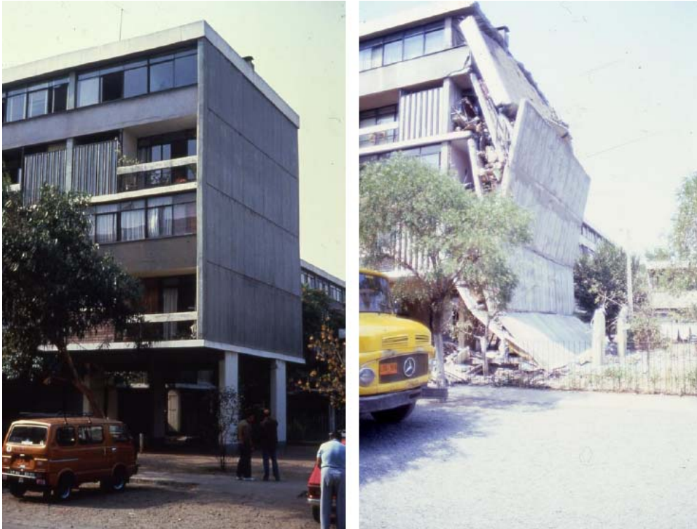
Figure A5. Villa Olimpica Buildings in Santiago. Twin buildings one of them partially collapsed. Note the initiation of the same type of failure at the top of the far column of the ground floor in the left side picture.
