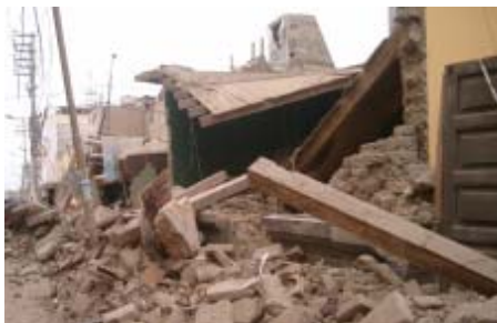
Figure 3. Collapse of roof
