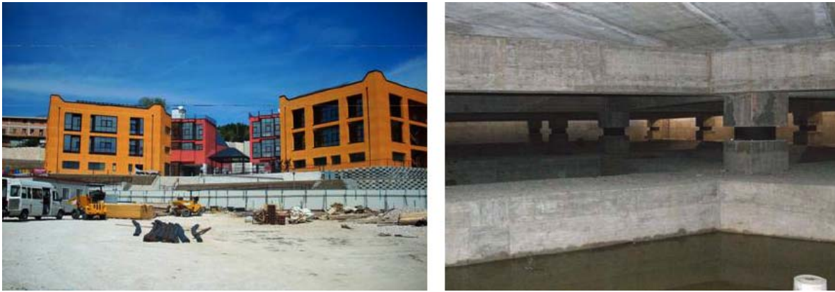
Figure 15. The new Francesco Jovine primary school and Le Tre Torri Professional and University Centre, erected in San Giuliano di Puglia (seismic zone 2 since 2003) on an unique seismically isolated slab, and its SI system (61 HDRBs and 12 SDs) during construction. The isolators were donated by the Italian ALGA, FIP Industriale and TIS manufacturing companies, SI design by a team of experts coordinated by the GLIS and ASS/ISi member P. Clemente of ENEA and tests by the University of Basilicata. Safety was certified by A. Martelli and the GLIS member C. Pasquale in September 2008
