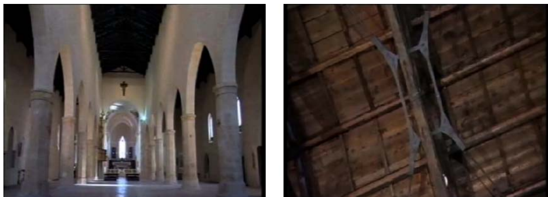
Figure 25. Internals of the Cathedral of Santa Maria di Collemaggio at L’Aquila (Figure 8) prior to the 2009 Abruzzo earthquake and view of one of the EPDs which had been installed on the roof at the beginning of the years 2000s to prevent overturning of the façade.
