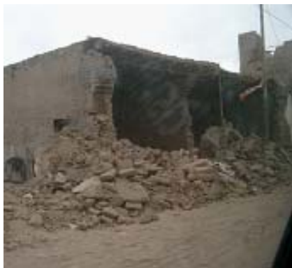
Figure 1. Overturning of walls
