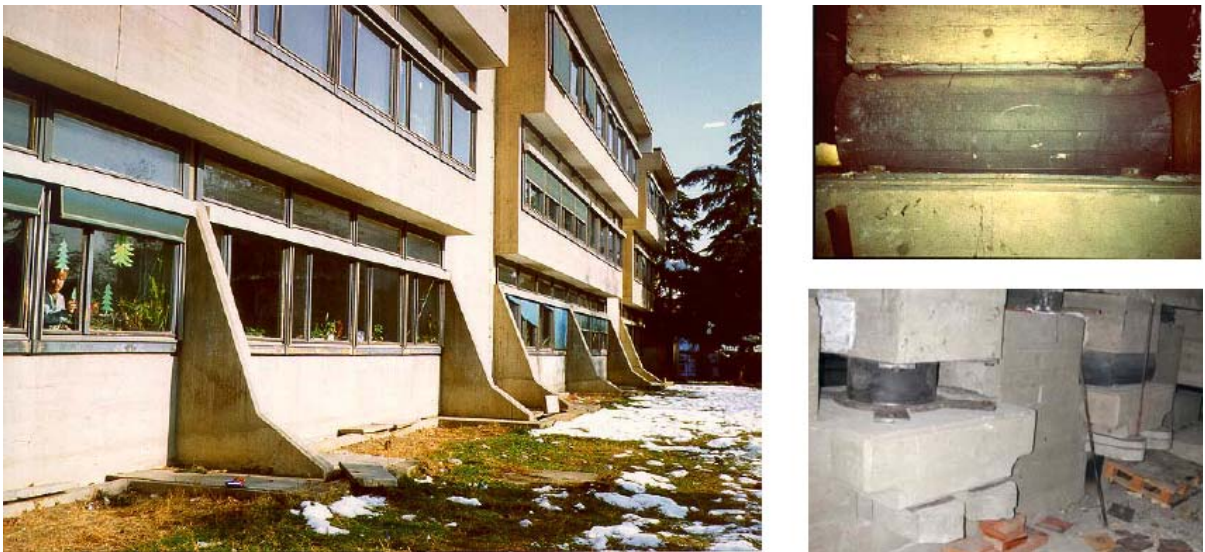
Figure 33. The isolated Pestalozzi school at Skopje (Macedonia), erected in the years 1960s, a very degraded original Low Damping Rubber Bearing (LDRB) and a new HDRB, close to not yet replaced original LDRBs
