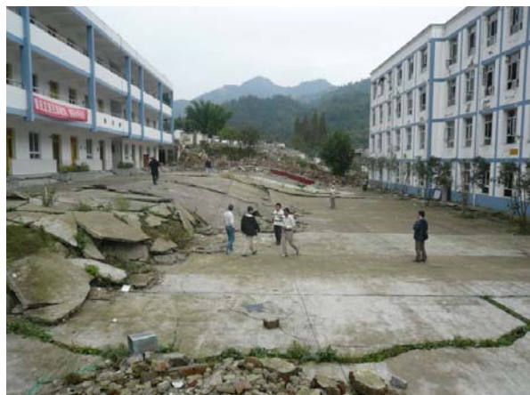
Figure 19. The left-side school building driven up 2 meters by the fault in Bailu (2008 ©T. Imamura)
