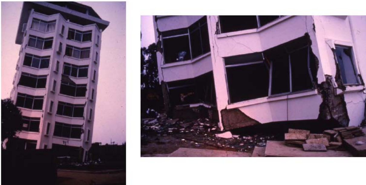
Figure A6. El Faro Building in Vina del Mar (Renaca). Shear wall failure at Ground floor due to significant torsion effects. Building was significantly inclined and was demolished soon after the earthquake.
