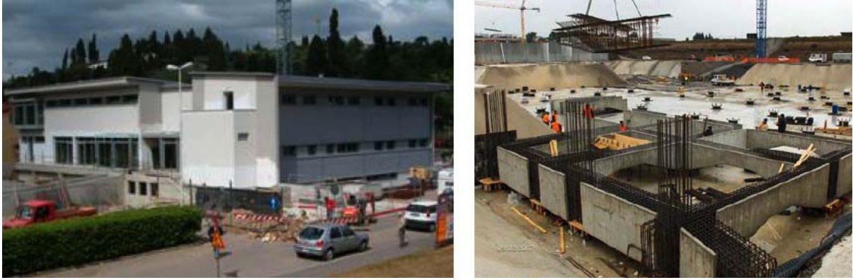
Figure 20. Left: Headquarters of the association Fratellanza Popolare – Croce d’Oro in Grassina (Florence), in seismic zone 2, isolated by means of SDs and Viscous Dampers (VDs); it is a L-shaped building to be used for civil defense certified as safe by A. Martelli in 2007. Right: NATO Centre of South Naples, in seismic zone 2 (399 HDRBs and ~20 dissipative SDs), during construction in 2007.
