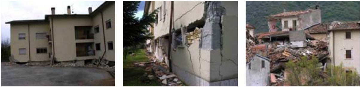
Figure 11. L'Aquila (April 2009): partly collapsed and heavily damaged private buildings
