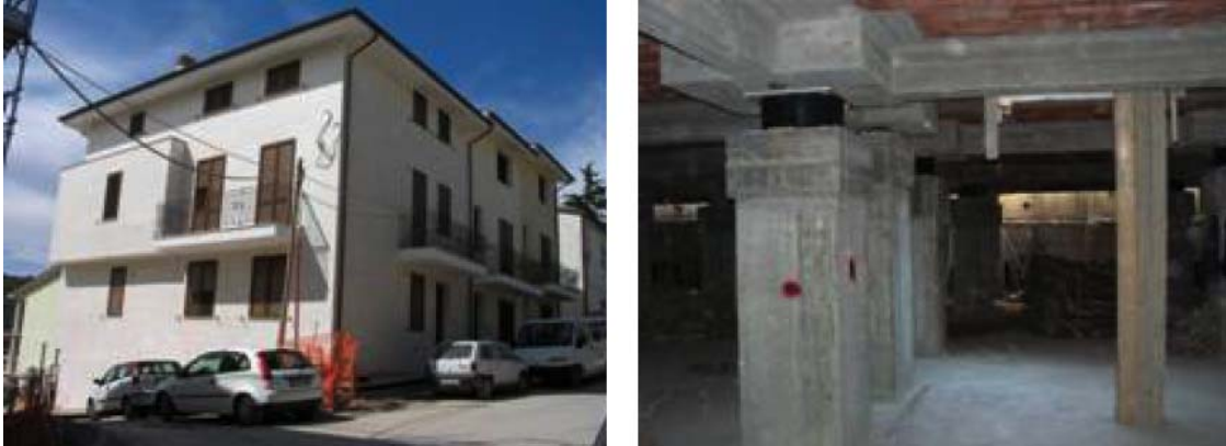
Figure 23. Left: dwelling building in San Giuliano di Puglia, isolated by 13 HDRBs and 2 SDs with the collaboration of ENEA, completed in 2007. Right: SI formed by LRBs and SDs of an 8-storey building under construction at Messina, in seismic zone 1 (its safety will be certified by A. Martelli)
