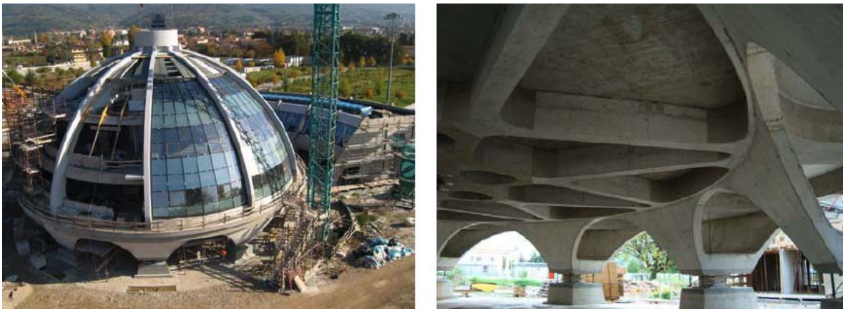
Figure 14. The main building (being erected on 10 HDRBs of 1 m diameter, see 2 of them on the right, covered provisional protections) and the adjacent service building (isolated by HDRBs and steel-PTFE Sliding Devices or SDs) of the Emergency and Management Operative Centre of the new Civil Defense Centre of Central Italy in Foligno (Perugia). Their safety will be certified by A. Martelli. The Foligno Centre will be formed by at least 7 isolated buildings (3 of them have already been completed). Its site was reclassified from seismic category 2 to seismic zone 1 in 2003, but no design changes of the structures and foundations were necessary, thanks to SI (an increase of the diameters of isolators was sufficient, as demonstrated by a study performed by ENEA)
