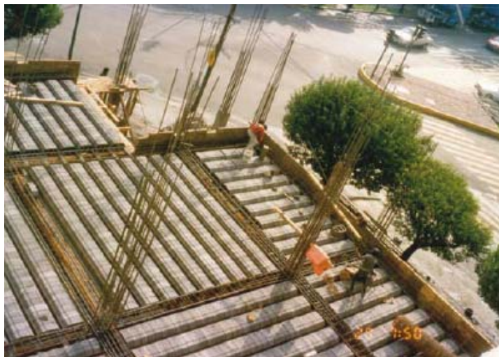
Figure 8. Engineered multifamily urban dwelling, based on prefabricated slabs, concrete beams and columns. Cost range 200 - 330 USD/m 2
