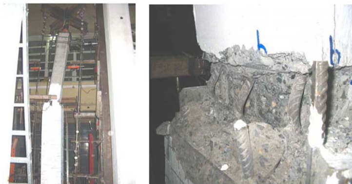
Figure 24. Damages observed in partially jacketed columns
