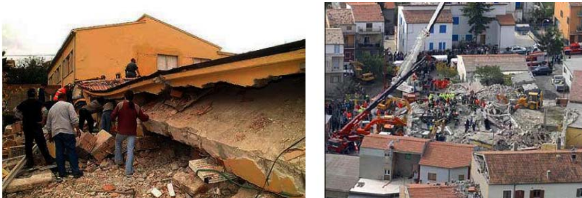
Figure 3. Collapse of the Francesco Jovine primary school of San Giuliano di Puglia (Campobasso) during the 2002 Molise and Puglia earthquake and search of survivors amid the debris
