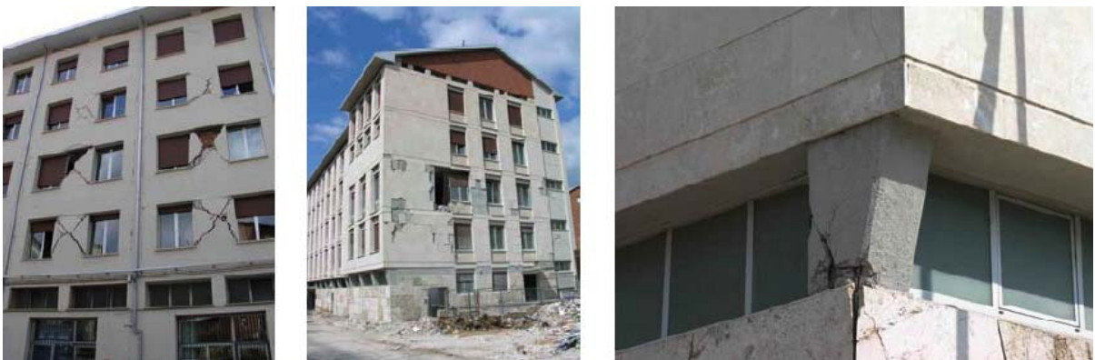
Figure 12. L'Aquila (April 2009): headquarters of ANAS (the Italian Agency for roads construction and maintenance), which suffered mainly non-structural damage (with the exception of two pillars, which, however, are repairable – see right) and might be retrofitted by means of SI
