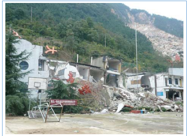
Figure 25 Collapsed elementary school buildings in Beichuan (© 2008 T. Imamura)
