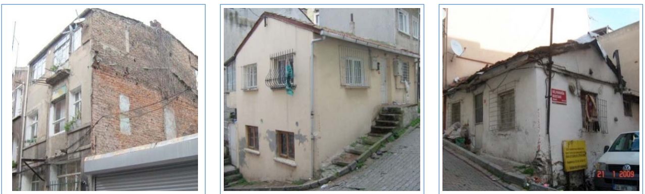
Figure 12 Typical non-engineered buildings in Turkey (Photos by Istanbul Culture University-Istanbul Technical University, Turkey)
