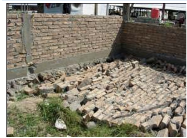
Figure 8 Wall collapse before completion
