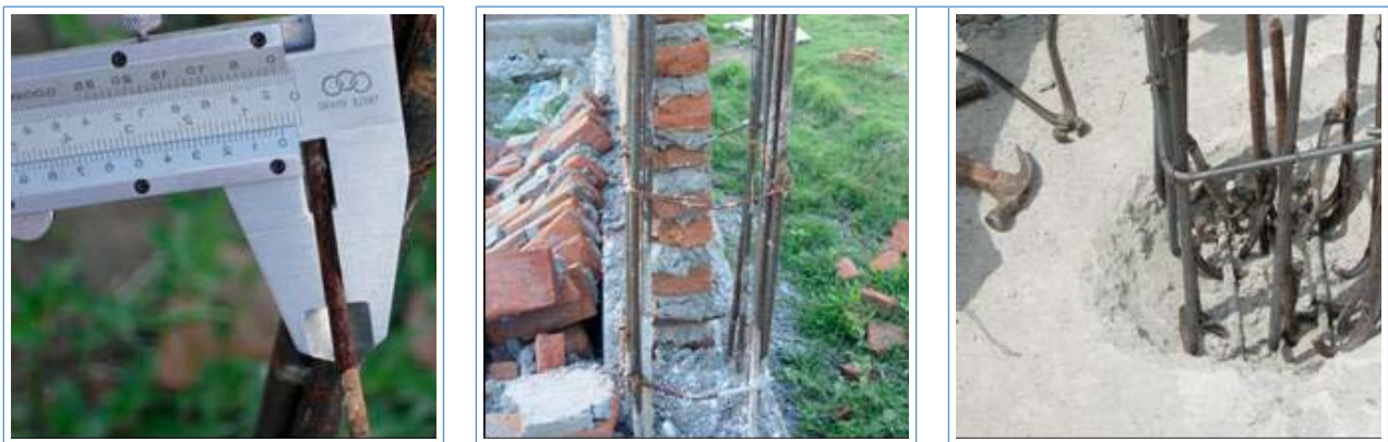
Figure 5 The use of a 4 mm stirrup (left), large spacing of stirrups (centre) and no seismic hook (right)
