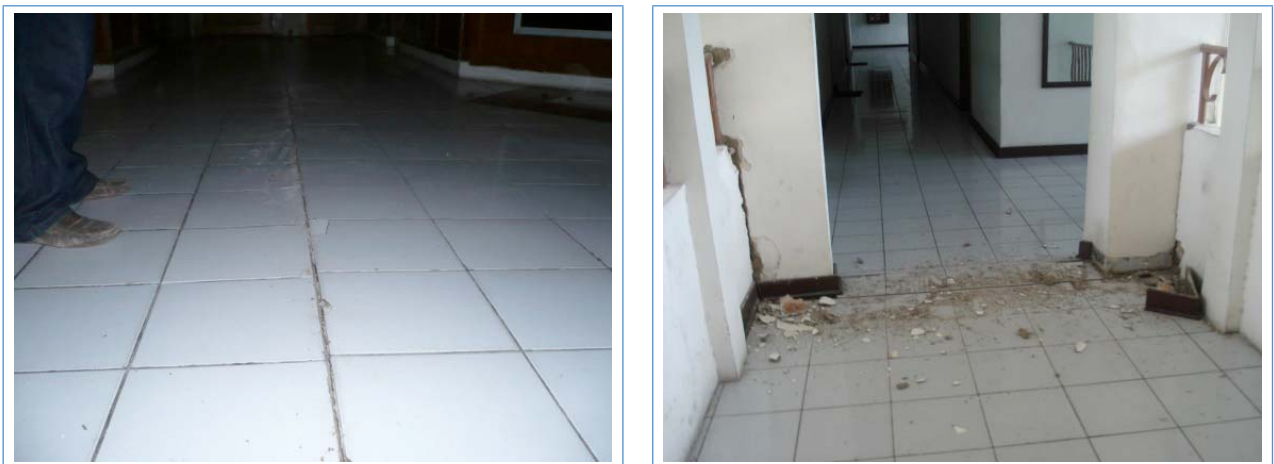
Figure 2 Damage to floors
