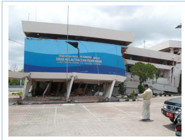
Figure 9 Damage to buildings due to the soft-storey mechanism
