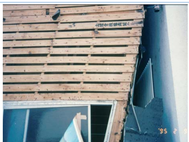
(b) Detail of damaged wooden house (Japan)
