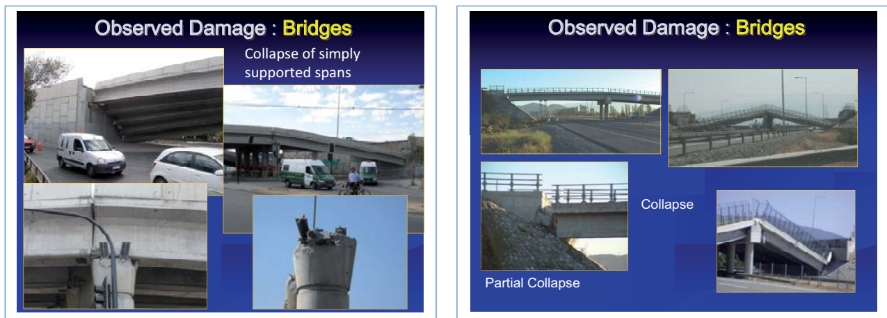
Figure 18 Bridge failure due to weak anchoring and lack of lateral support
