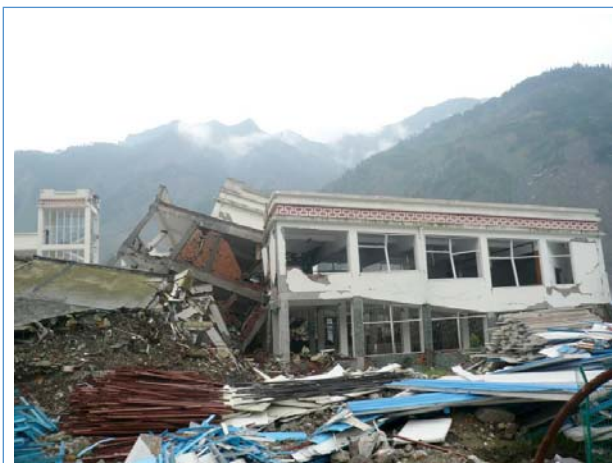
Figure 22 Collapsed junior high school buildings in Yingxiu (© 2008 T. Imamura)
