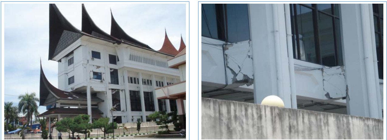
Figure 10 Damage to beams
