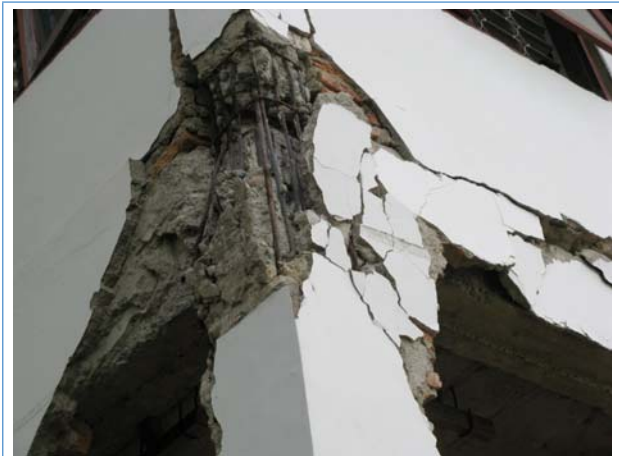
(b) Strong beam/weak column failure exacerbated by poor detail and quality (Food Security Agency Building)
