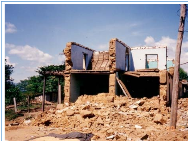
(a) Damaged tapial house (Peru)
