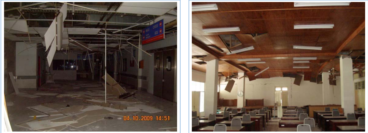
Figure 5 Damage to ceilings
