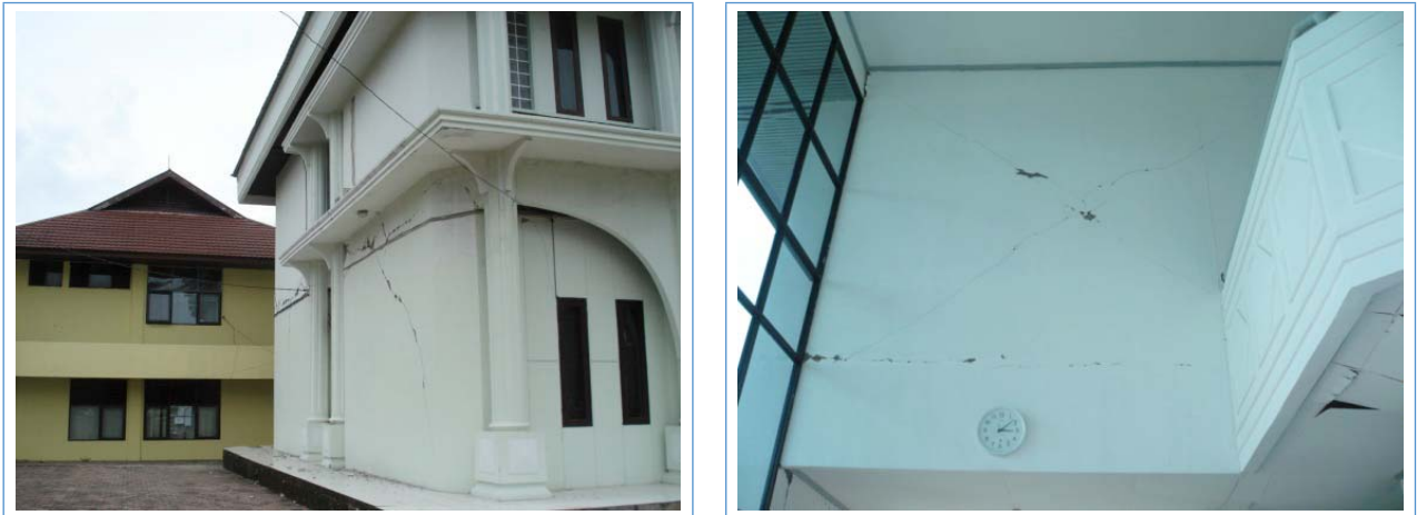
Figure 1 Damage to partition walls
