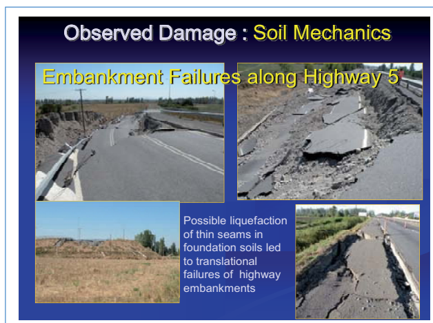
Figure 22 Soil failure and landslides on the embankment of Highway 5
