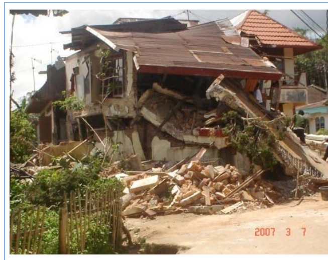
Figure 1 One of the collapsed houses in the research
