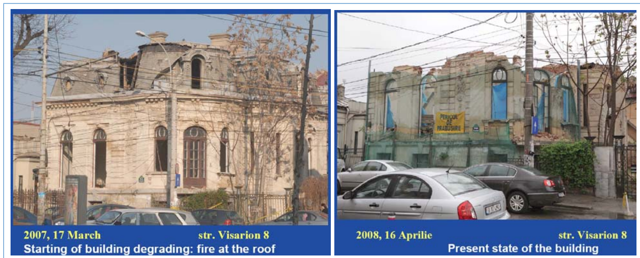
Figure 14 A Bucharest heritage building in the city centre, intentionally prepared for demolition
