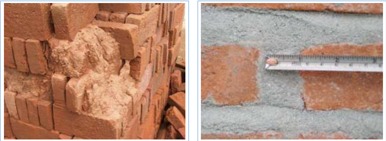
Figure 6 Melting bricks (left) and large brick spacing (right)
