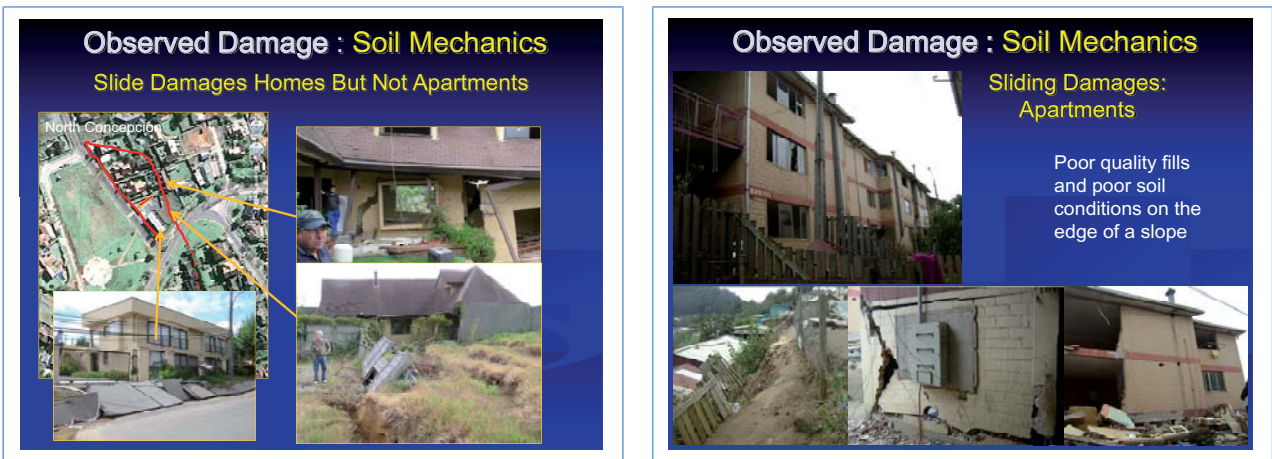
Figure 20 Failure of houses and small buildings due to landslides and poor soil conditions
