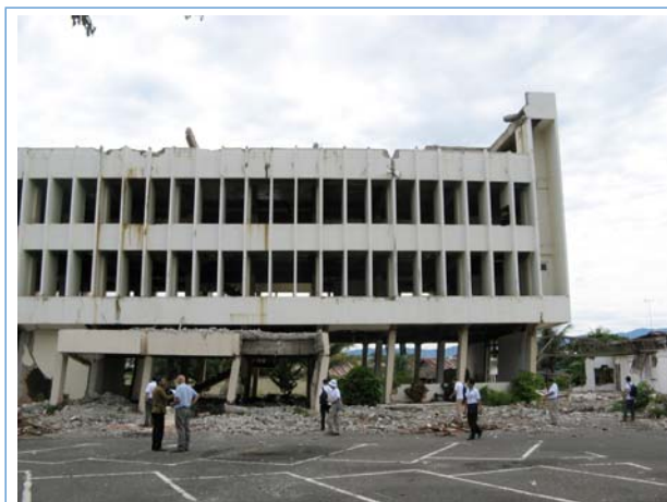
(a) Soft-storey failure exacerbated by liquefaction (Provincial Public Works Office)
