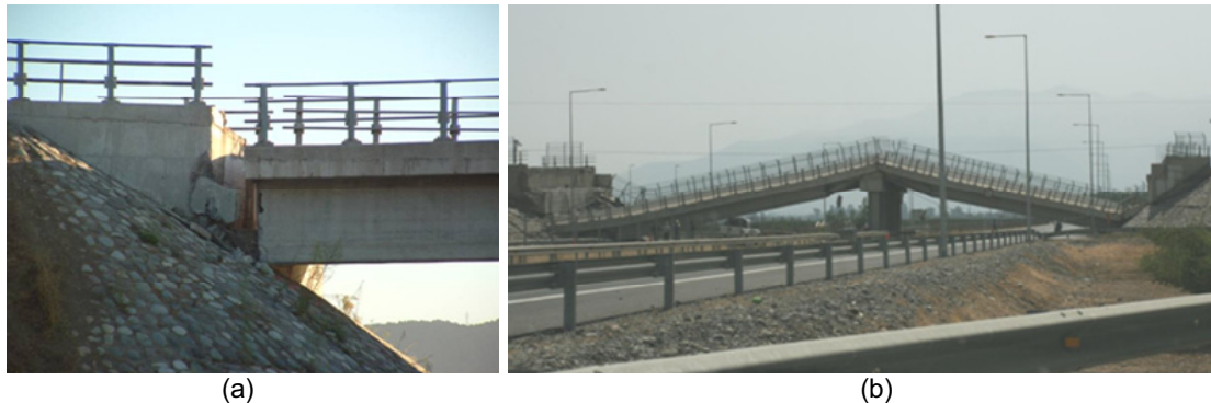
Figure 8. (a) Partial collapse of the superstructure, (b) total collapse of the superstructure. All photographs were taken at Ruta 5 Highway
