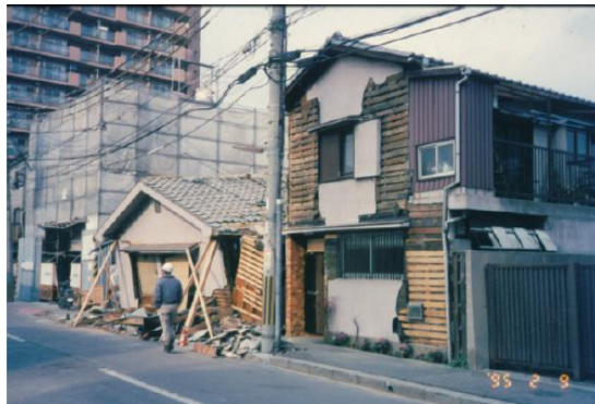
(a) Damage concentrated to the first storey
