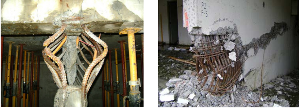
Figure 11. Typical compression failure of heavily loaded thin walls
