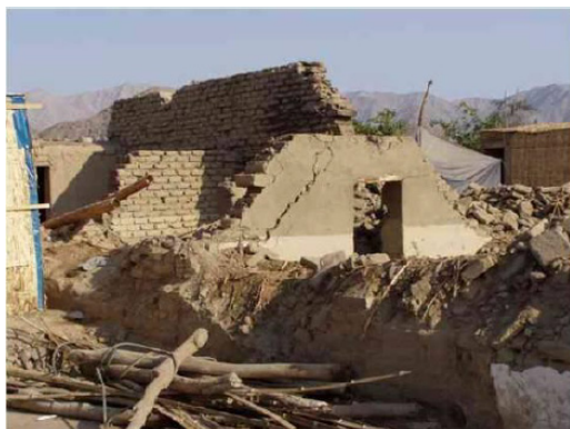
(a) Damaged adobe (2007 Pisco Earthquake)
