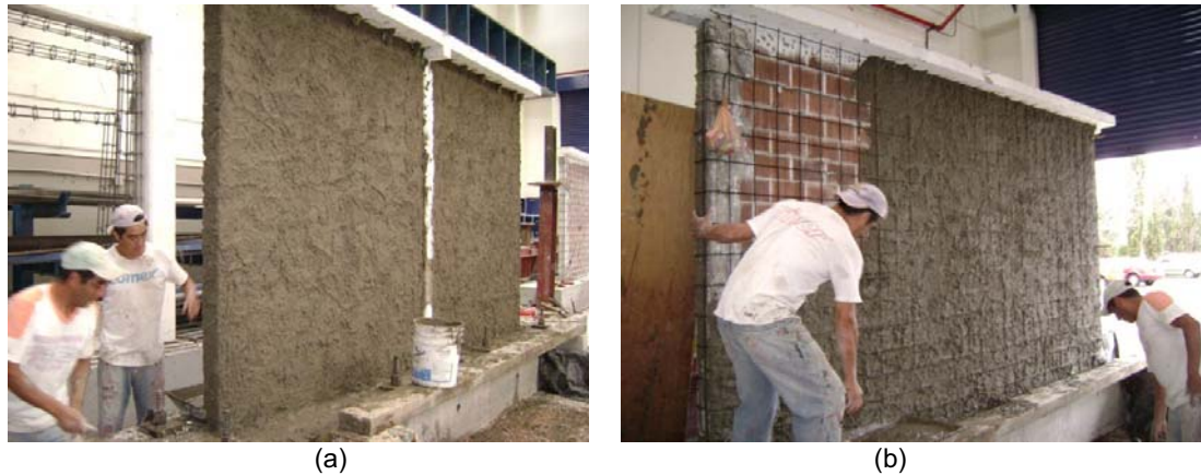
Figure 7. Confined ceramic masonry walls with different type of retrofitting procedures: A) Mortar with steel fiber; B) Mortar with wire mesh as examples of current experiments
