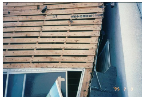
(b) Detail of the damaged wooden house
