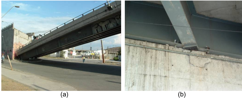
Figure 11. Bridge in Matta Av.: (a) collapsed span, (b) support at the abutment
