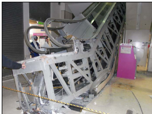
Figure 33. An escalator fallen down at the Sendai-Saiwaicho shopping center (Sendai city)
