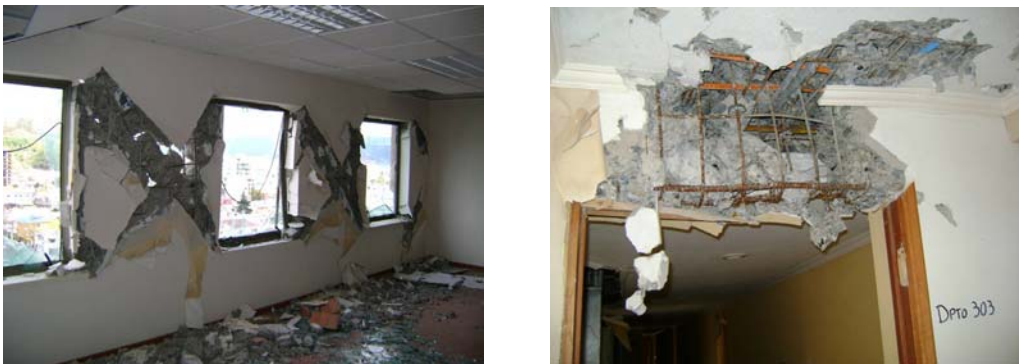
Figure 6. Typical failure of short columns and coupling beams
