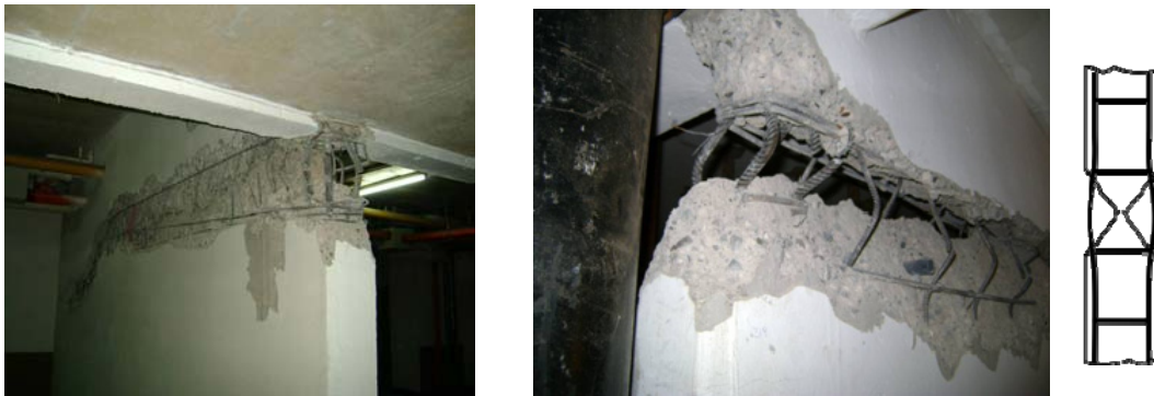
Figure 9. Typical compression failure of heavily loaded thin walls
