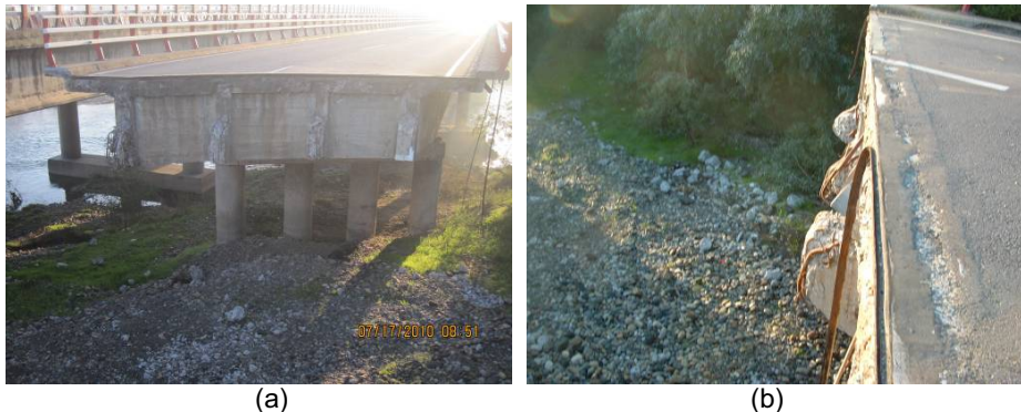
Figure 12. Nebuco Bridge: (a) collapsed span, (b) support of collapsed span
