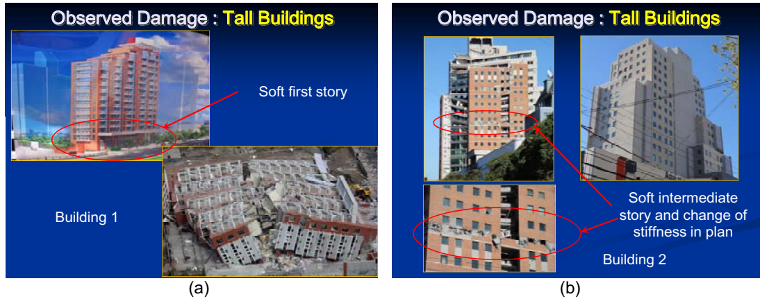
Figure 4. (a) Collapsed building with soft first story, (b) Building with partially collapsed soft intermediate story.
