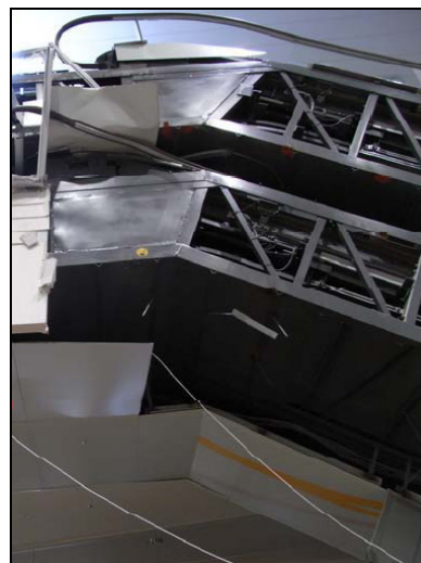
Figure 34. Escalators stuck together at the Izumi-osawa shopping center (Sendai city)
