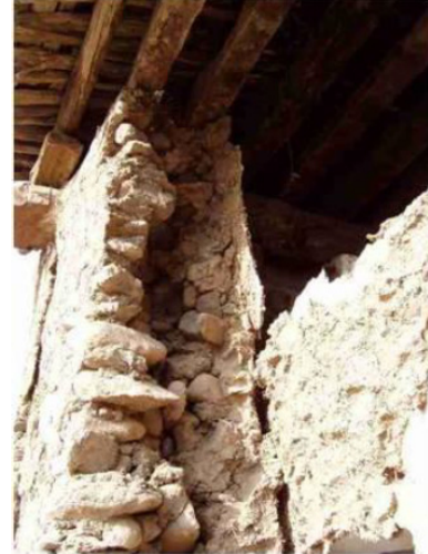
(b) Damage to the stone masonry wall
