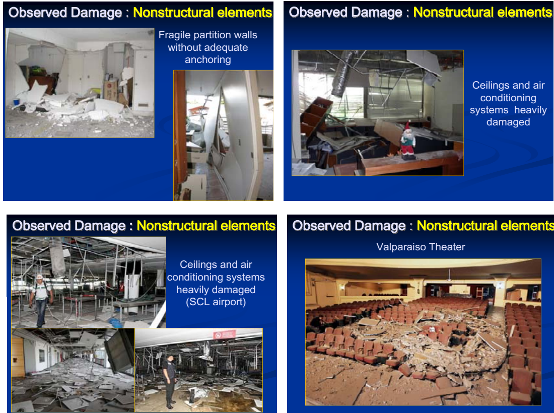
Figure 7. Typical damages in non-structural elements.
