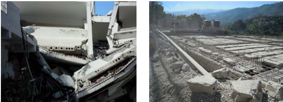
Figure 1. Lightweight elements used in floor systems without reinforcement. In the right side photo it is clear the lack of reinforcement in the wall – slab joint, these procedure do not allow the coupling of vertical elements to withstand seismic demands
