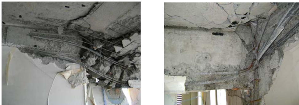
Figure 12. Poor anchorage of beam reinforcement in thin walls
