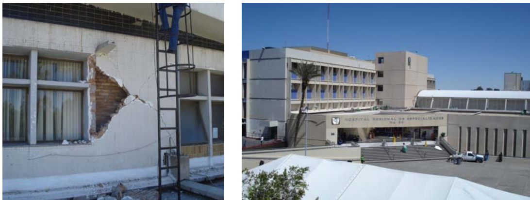
Figure 5. Hospital temporarily closed due to non-structural damage
