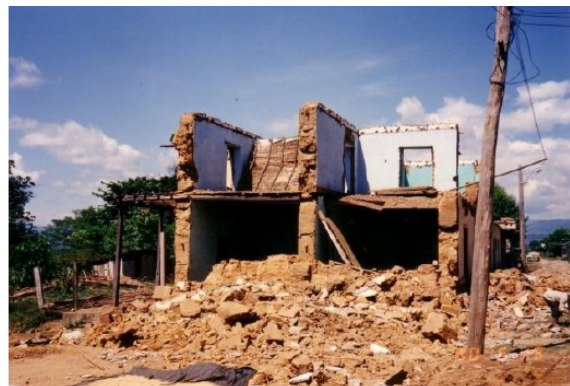
(b) Damaged tapial (1990 Rioja Earthquake)
