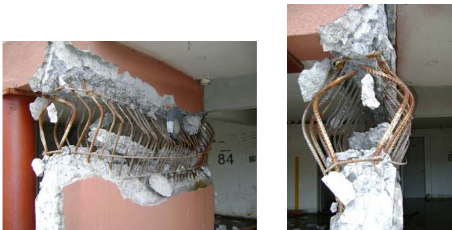
Figure 10. Typical compression failure of heavily loaded thin walls
