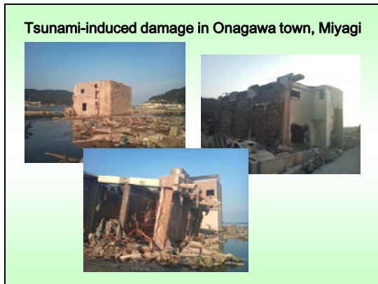
Figure 23. Tsunami-induced damage in Onagawa town, Miyagi (2011 ©T. Imamura)
