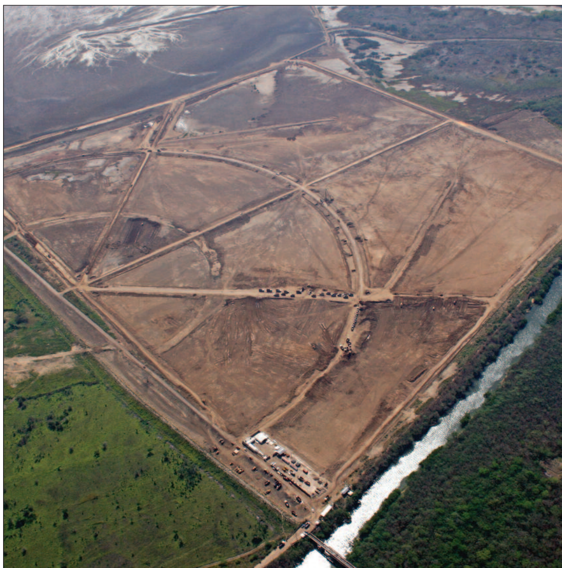
Soapberry Sewerage Plant, Kingston
