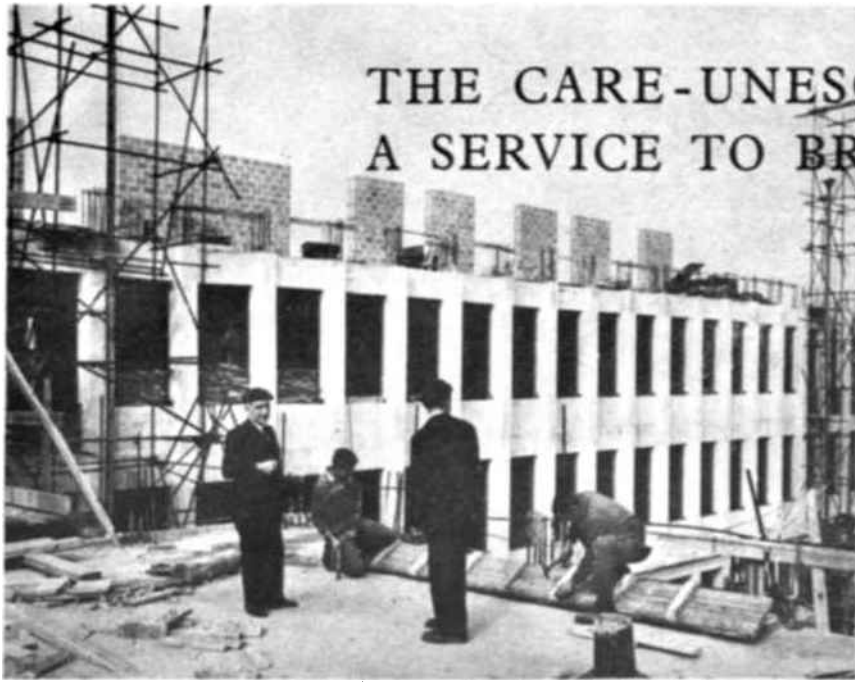
Six years after the entire University of Caen was destroyed during the Allied advance through Normandy, University Rector, Pierre Daure (extreme left) watches the construction of the first new building. The University's temporary library, housed in a former school, recently received a consignment of CARE-UNESCO books donated through the help of the War Dads Auxiliary of Kansas City, Missouri.
