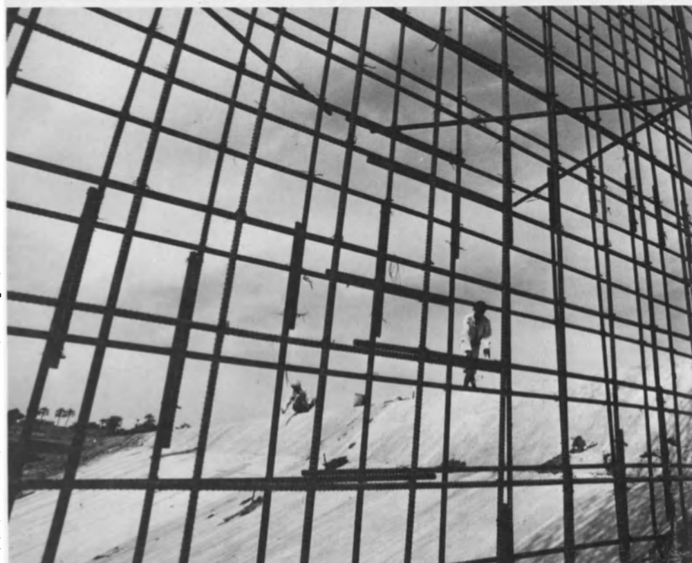
Work in progress on a weir which forms part of a project for the improvement of the surface water irrigation system at Wadi Zabid, Yemen Arab Republic. The project, financed with the help of a 10.9 million dollar credit from the International Development Association (IDA), was completed in 1979 and covers some 17,000 hectares.
