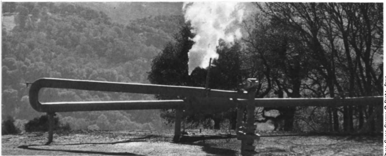
Hot water geyser being tapped for geothermal energy.
