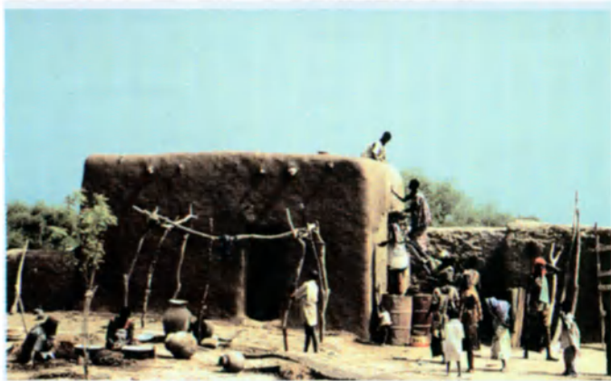
Kotoko women builders of northern Cameroon renovate a cob-walled dwelling and teach their skills to young apprentices.
