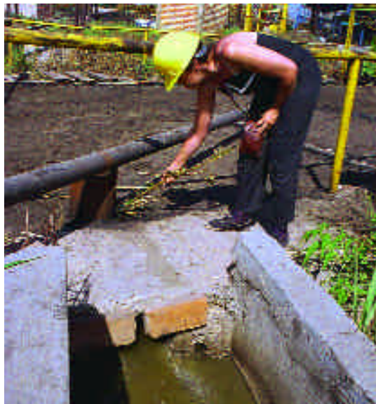
Mending an antiquated installation.
