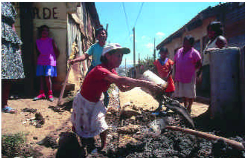
A community project to build underground sewerage and drinking-water installations in Guatemala City.
