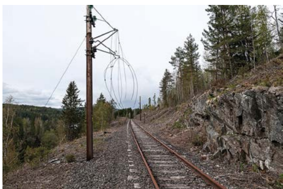
The overhead line equipment on the Tinnoset Line is largely gone due to theft. Photo: Per Berntsen.
