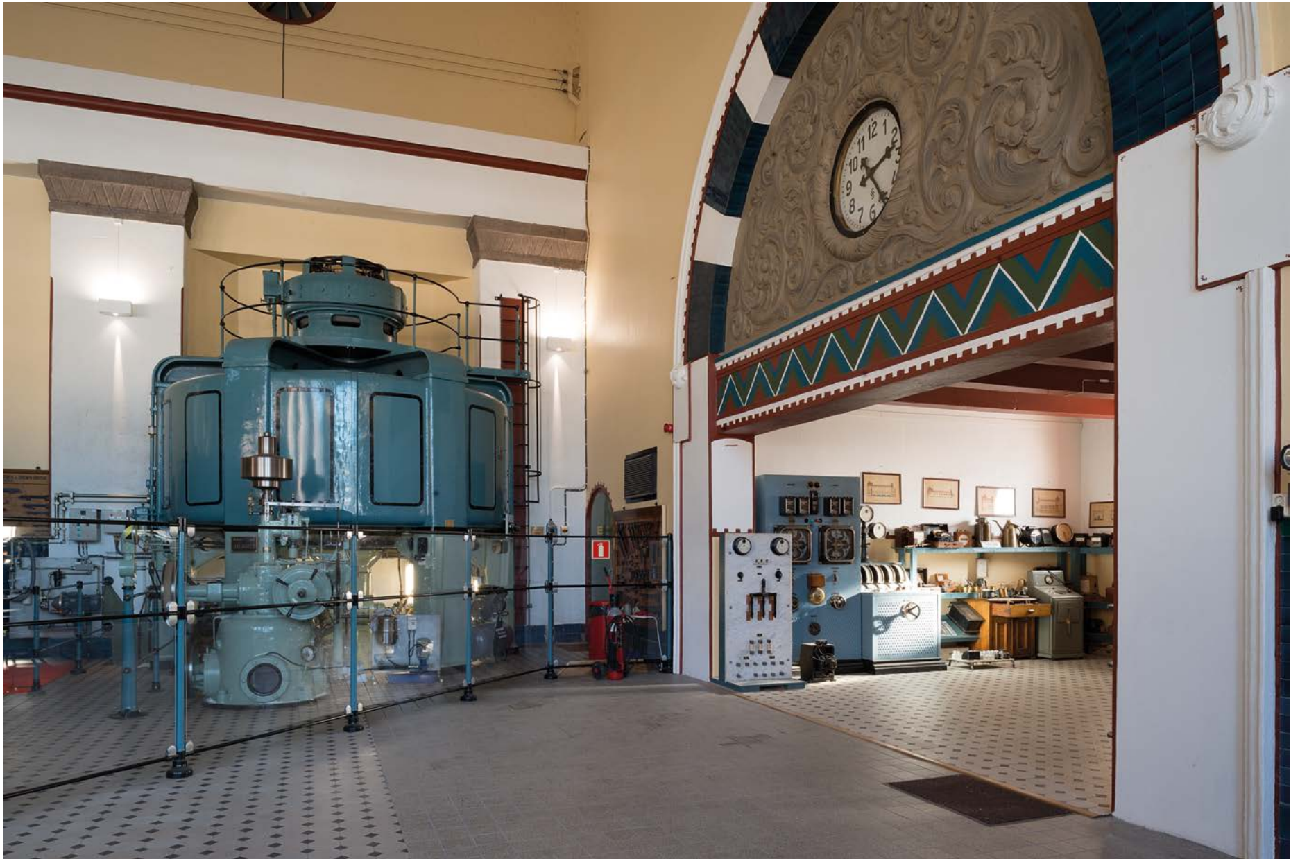
Fig. 13 Tinfos II Power Plant. Photo: Per Berntsen
