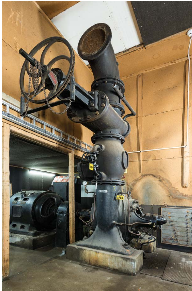
Fig. 62 AEG Pump in Pump House, Hydro Industrial Park in Rjukan. Photo: Per Berntsen
