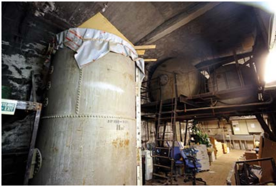
The tanks in the Hydrogen Plant. Photo: Eystein M. Andersen
