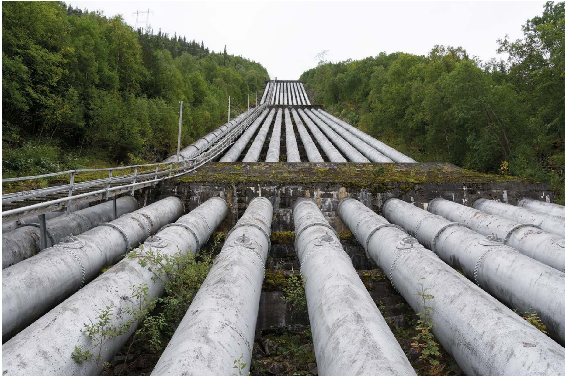
Fig. 21 Penstock at Vemork Power Plant. Photo: Per Berntsen
