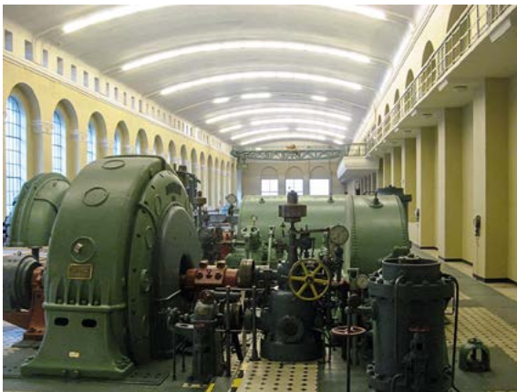
Interior of Såheim power Plant. Photo: Trond Taugbøl.
