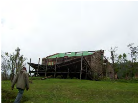
Hurricane Dean damage to Cabin 1 at Holywell
