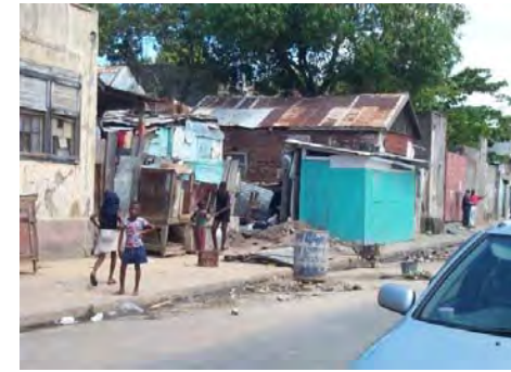
A number of houses in KSA are in a state of disrepair and cannot be reasonably renovated.
