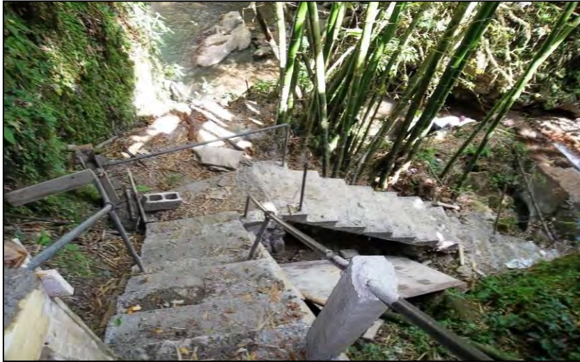
Construction of stairs down to Nanny Falls for safety and improved access
