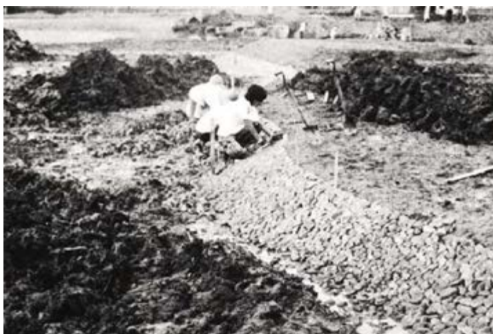
photo A4-70 Repaired state of north shore of the pond. ©Hiraizumi Town Board of Education
