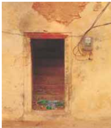
Deteriorating fabric and evidence of poor maintenance
