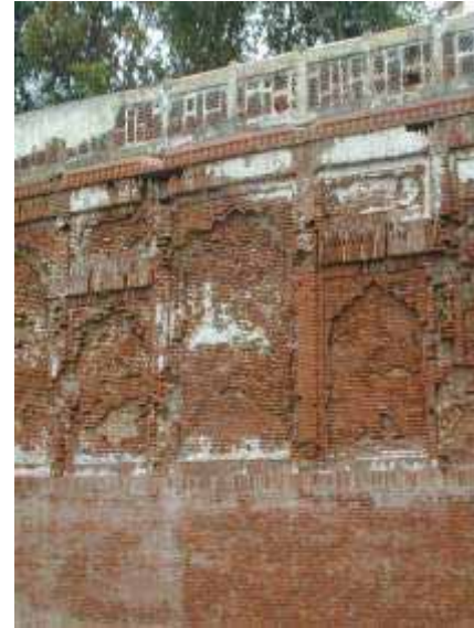
Eroding decorative brickwork of the Perimeter Wall in need of conservation
