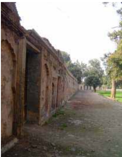
Internal face of the west Perimeter Wall showing bulging
