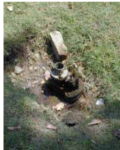
Poorly maintained valves for watering the gardens
