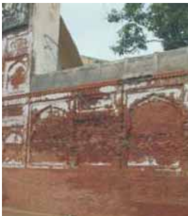
Deterioration of the brick of the perimeter wall
