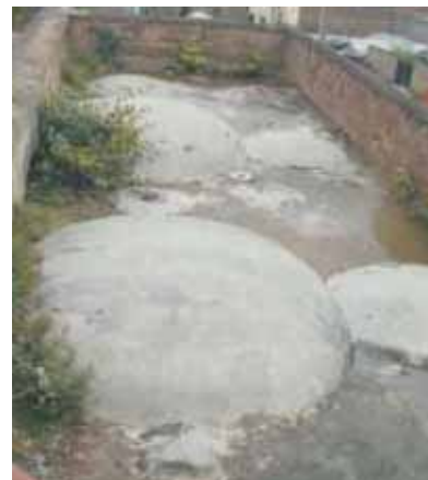
Roofs of buildings in need of maintenance
