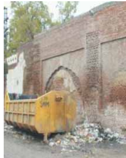
Uncontrolled garbage collection against the wall of the site
