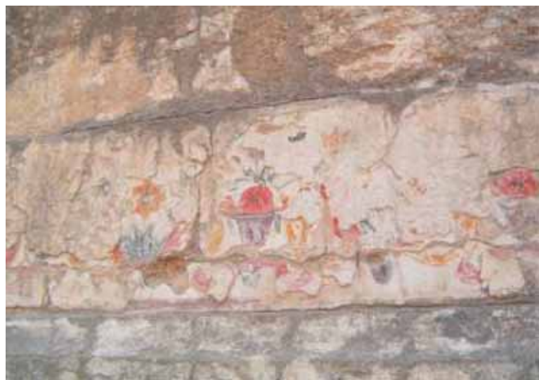
Exposed fresco work on exterior of the Perimeter Wall in need of conservation
