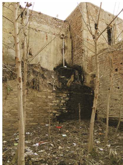
Sewerage being disposed off through the wall
