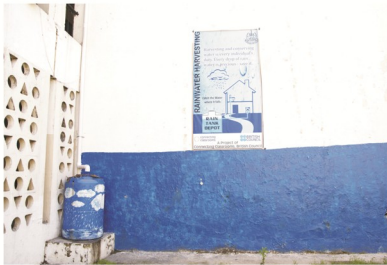
Harvested water being supplied into toilets
