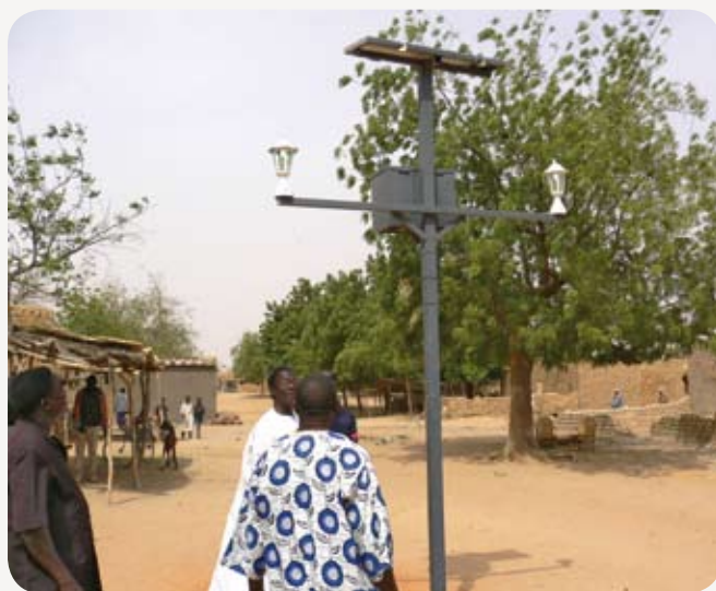
Village square in Burkina Faso equipped with a solar street lamp.
