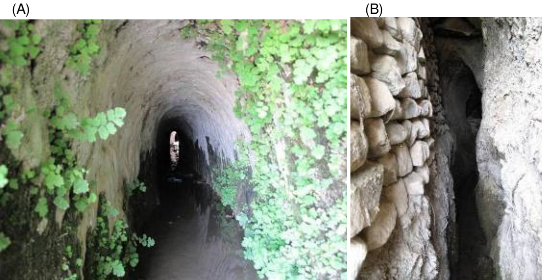
Figure 5. (A) Round arch karez tunnel in limestone at Zimzimuk; (B) Pitched and pointed arch Sarsula karez at Girdashekhal (in limestone). (Photos by Dale Lightfoot)
