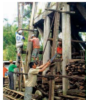
Rehabilitation of the roof of Oma Sebu (the Chief's House), Onohondro village, South Nias © ECO Unit
