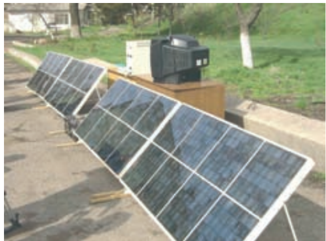
Solar energy panels, Uzbekistan
