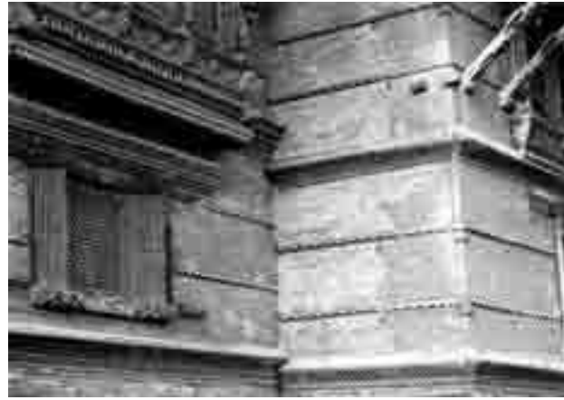
Fig. 92. Joints between new and old bricks.
