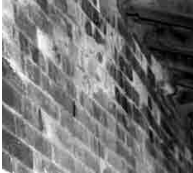
Fig. 89. Salt crystal on wall surface.
