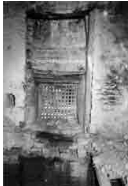
Fig. 43. Deterioration of timber elements from damp.
