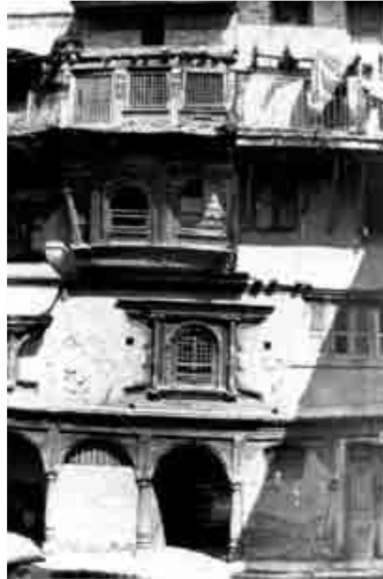
Fig. 55. Damage of carved elements.
