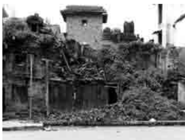
Fig. 41. Damage from water penetration.
