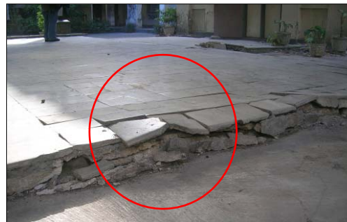
Fig. 174: Displaced tiles should be removed and the sand or soil under the floor should be stabilized
