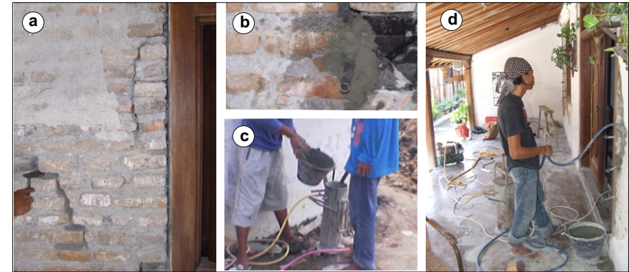
Fig. 180: Injection process: a. clean the crack from dirt, b. install a 3/4" pipe and cover with sealant adhesive, c. mix Portland cement with bonding agent and additive grouting, d. pour the modified cement into the crack using low-pressure injection system
