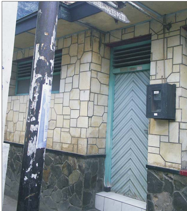
Fig. 151: Foundation wall (natural stone) which is above ground level Gbr. 151: Pelapis dinding pondasi (batu alam) yang terlihat di atas tanah
