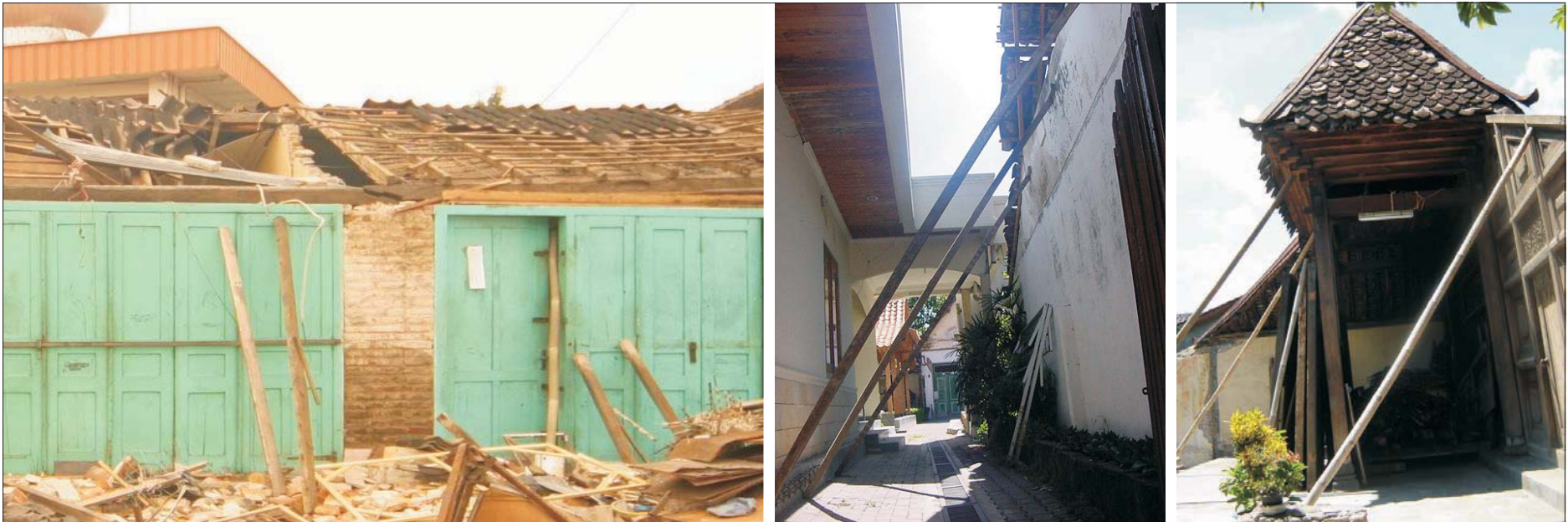
Fig. 168: Treatment of the broken or tilted wall that is supported by bamboo/wooden beam Gbr. 168: Pengamanan dinding yang miring disangga dengan bambu/kayu
