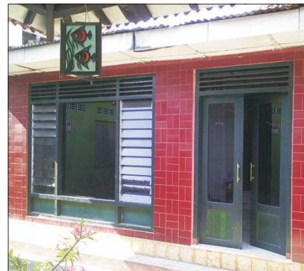
Fig. 154: Ceramic-layered wall is not recommended for use on facade Gbr. 154: Dinding dilapis keramik pada fasad tidak disarankan
