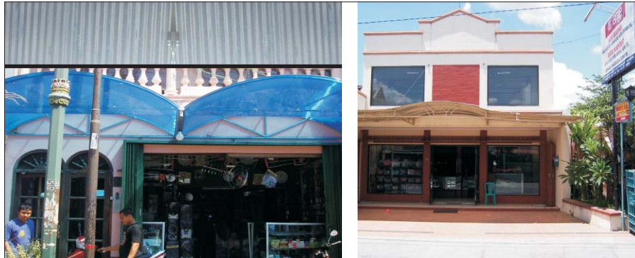
Fig. 156: Polycarbonate and zinc roofing are not recommended Gbr. 156: Atap polycarbonate dan seng tidak disarankan
