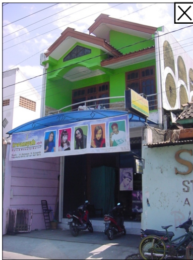
Fig. 159: Fiberglass is not recommended as a roof cover
