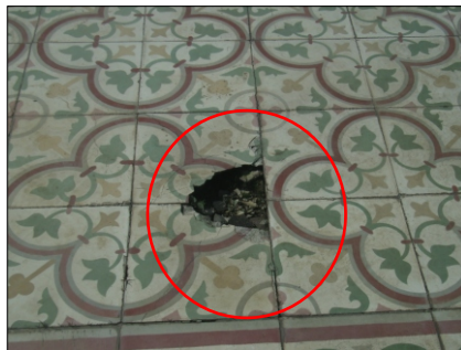
Fig. 173: Broken floor tiles need to be replaced with appropriate new ones
