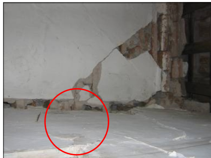
Fig. 172: Broken bligon floors should be repaired using a mixture of red cement, sand, and lime
