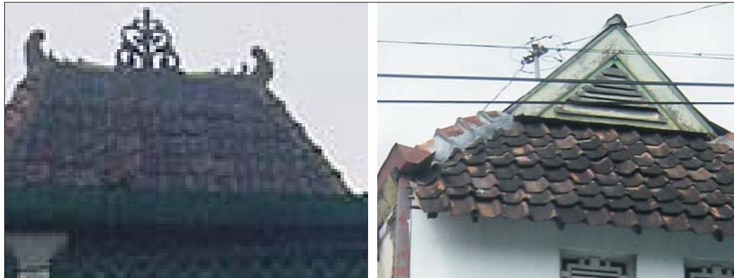
Fig. 96: Roof cover material and ornament of Kalang house, (a) makutha and (b) krepyak Gbr. 96: Bahan dan ornamen penutup atap rumah Kalang, (a) makutha dan (b) krepyak
