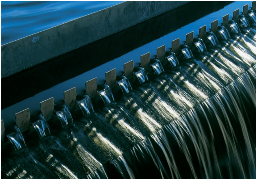
Fig. 3. La Farfana Water treatment plant.
