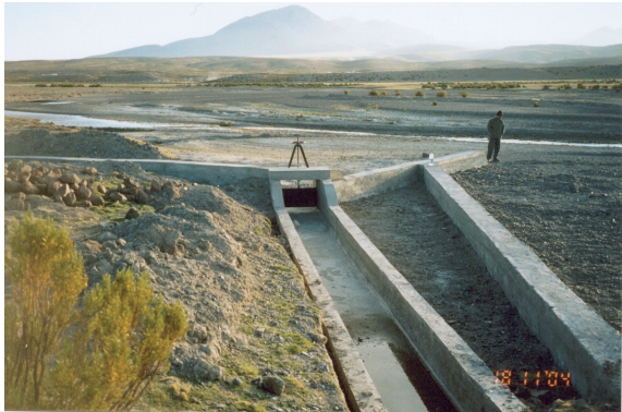
Figure 21. Water intake in Bocatoma River, Caquena
