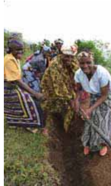
Local community installing water pipes for their village in Kinhare, Tanzania. This project will bring safe drinking water to the region for the first time. Previously people had to collect often unsafe drinking water from distant streams and carry it in buckets
