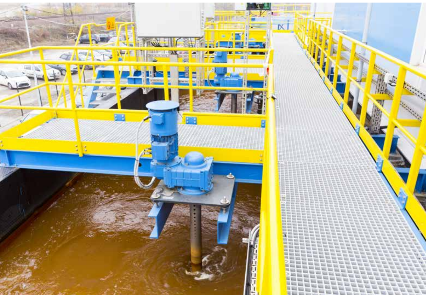
Rainwater treatment plant Photo: © Cylonphoto/Shutterstock.com
