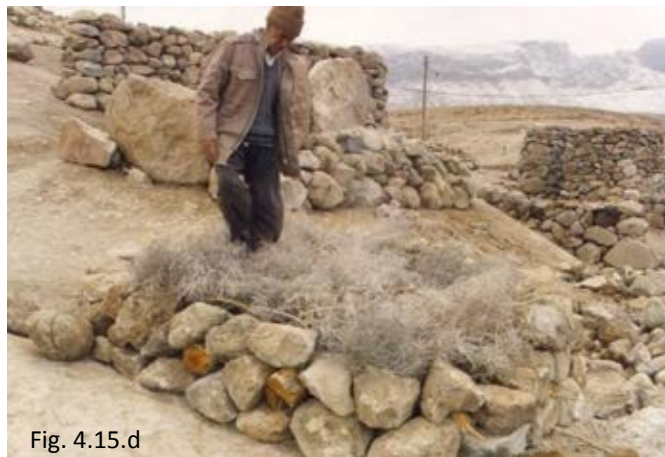
Fig.4.15a/e Different process of restoration of damaged roof 1381/2002
