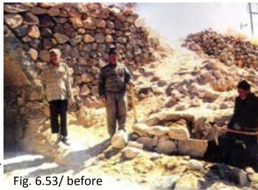
Fig. 6.53/56 Area next of old bath before and after conservation activities within 1381/2002 and 1384/2005
