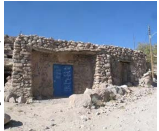
Fig.4.87: An inappropriate construction with troglodyte fabric of Maymand
