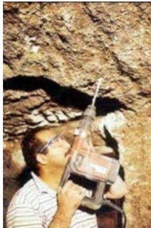
Fig.4.12 Consolidation damaged roofs 1380/2001
