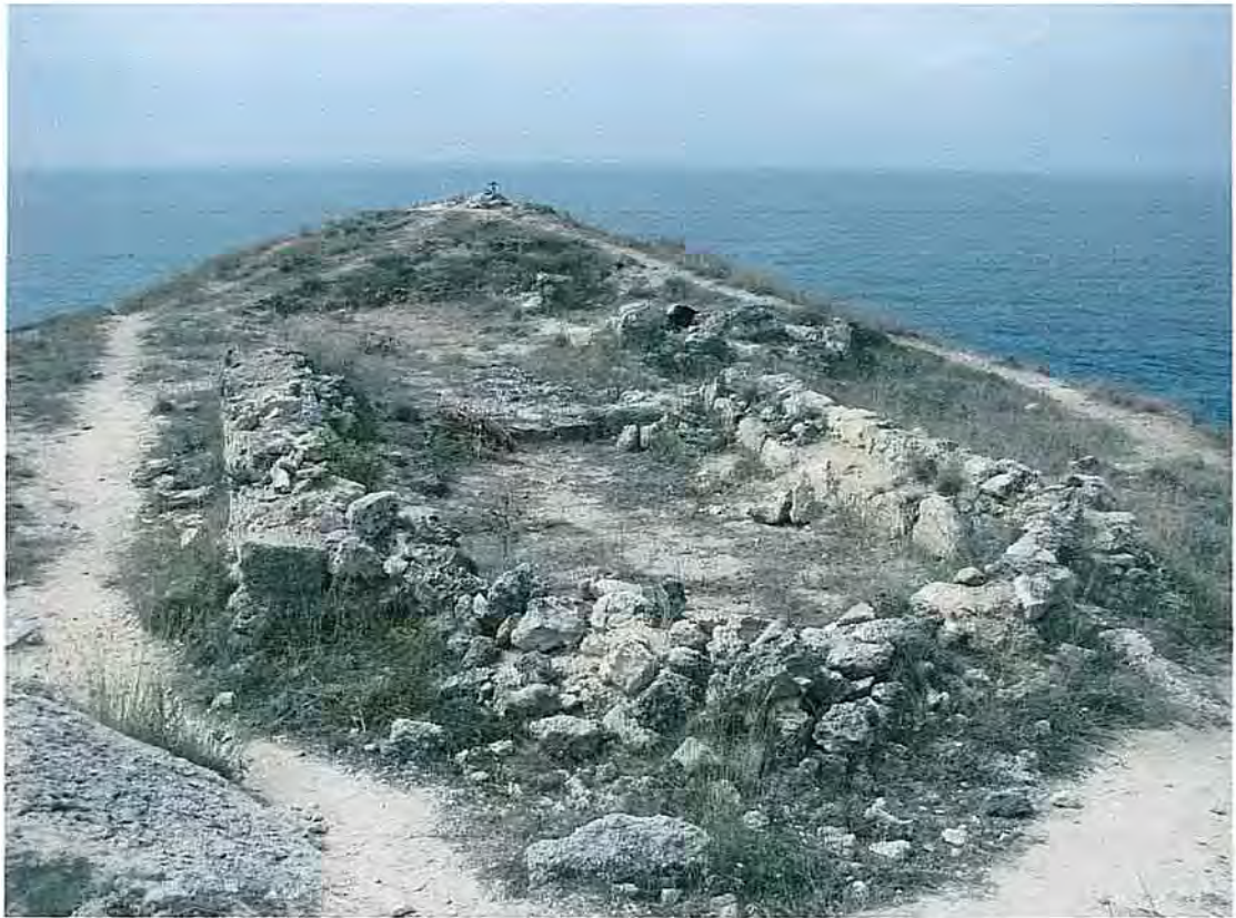
Fig. 25. Deteriorating ruins of a ground-based church on Cape Vinogradny 15 years after conservation
