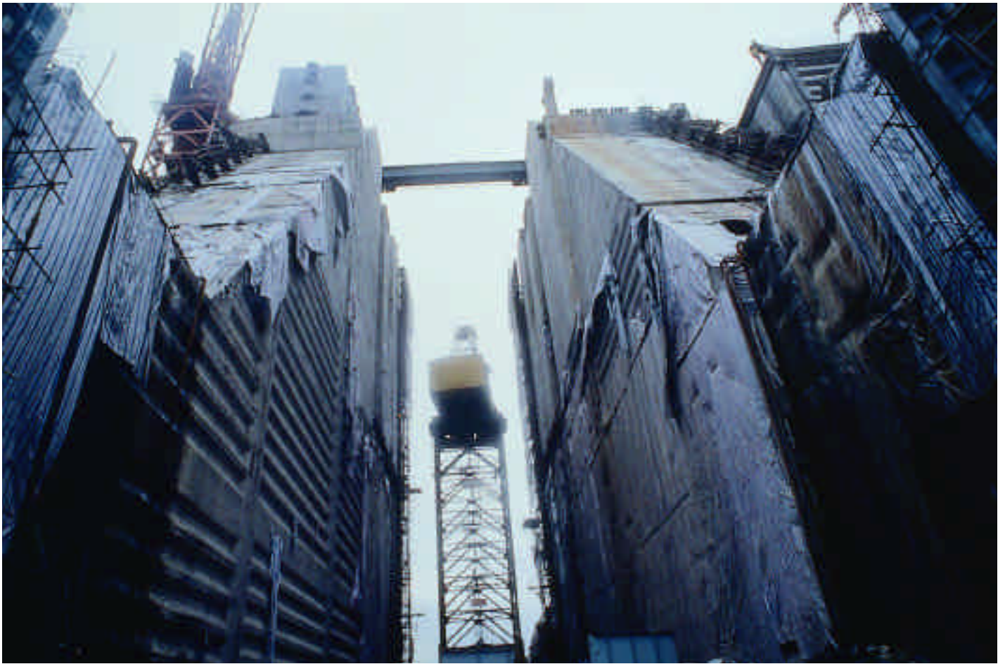
On the rise: construction of a dam as part of the giant Three Gorges project on China's Yangtze River.
