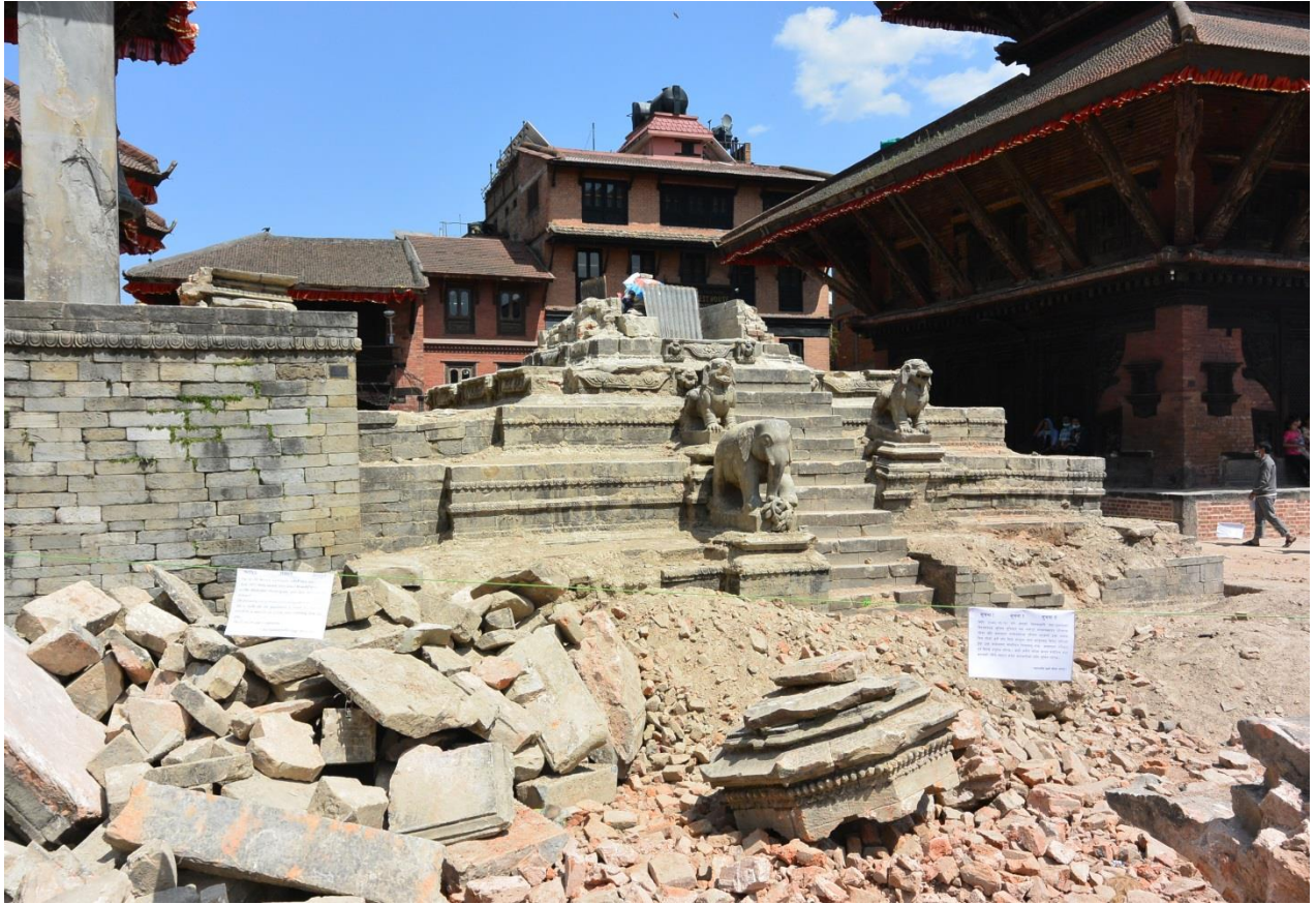
Photo: The earthquake damages monuments at Bhaktapur Durbar Square (c) UNESCO \D. Andolfatto
