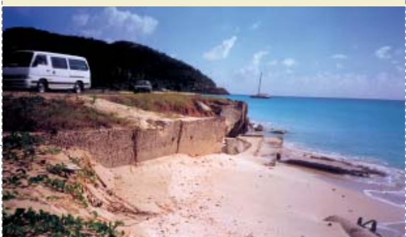
This coastal highway at Darkwood Beach in Antigua is frequently damaged during hurricanes, 2000
