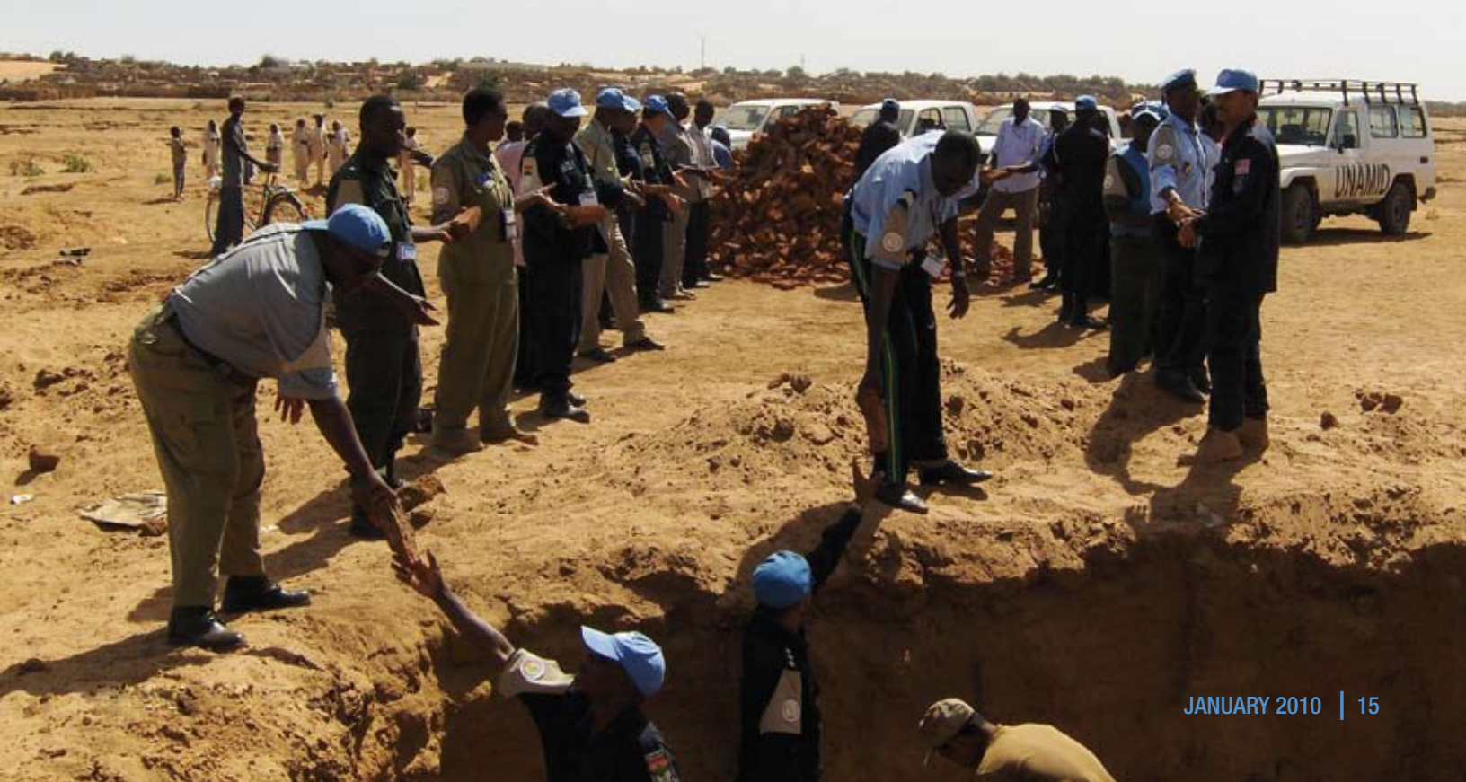
UNAMID police officers assist with the construction of a Community Policing Centre (CPC) near El Fashir, Darfur. (UNAMID Photo)
