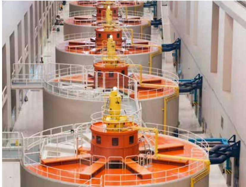
Hydroelectric power generators Photo: © iStock.com/leezsnow
