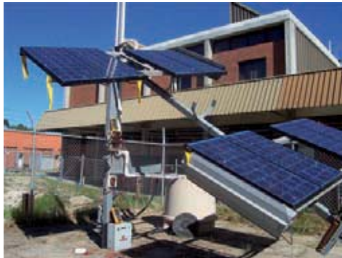
Construction last year of a prototype mini-grid hybrid power system blending solar, wind and micro-hydro energy generators with a conventional diesel generator. This system will supply local communities in Indonesia with power and clean water
