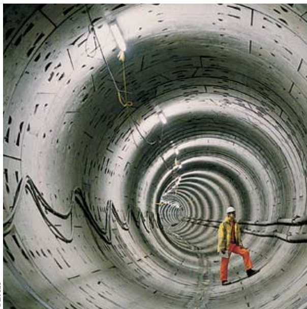
The application of a spray-applied membrane designed by BASF on the interior walls of a tunnel being built in the United Kingdom reduces the amount of concrete required, saving millions of euros in construction costs and reducing CO 2 emissions from cement-making.
