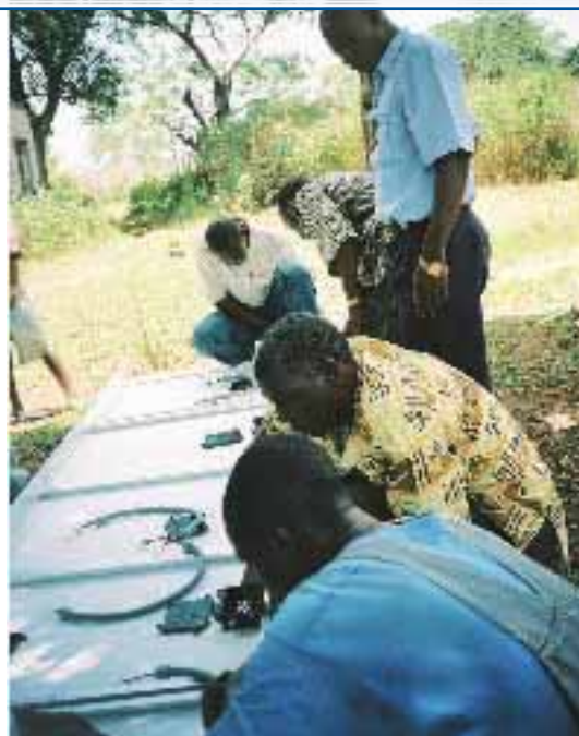
Electrical cabling of solar panels and the installation of solar systems by participants as part of practical field-work organized by UNESCO in Bamako (Mali) in 2003
