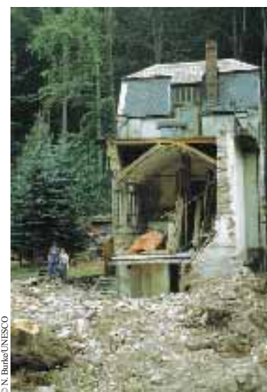
A house on the road to Prague (Czech Republic) after floods devastated Central Europe in August 2002
