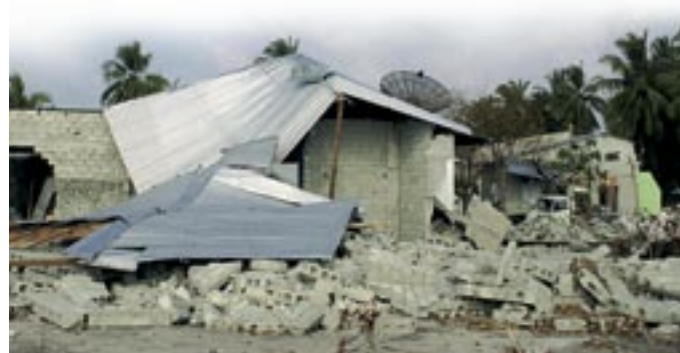
School buildings in the Maldives devastated by the tsunami. A new Coalition on Education is set about improving the safety of school buildings in a disaster (see p.8)
