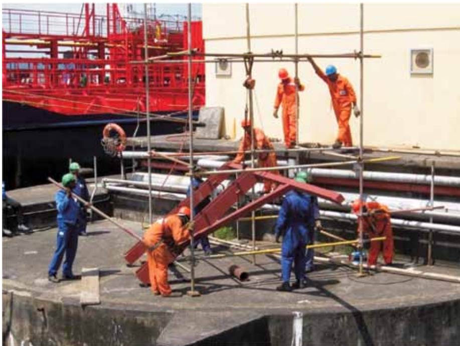
Figure 4. Installation of Tide Gauge at Port SONARA (photo credit: Frédéric Simon, 22 June 2008).
