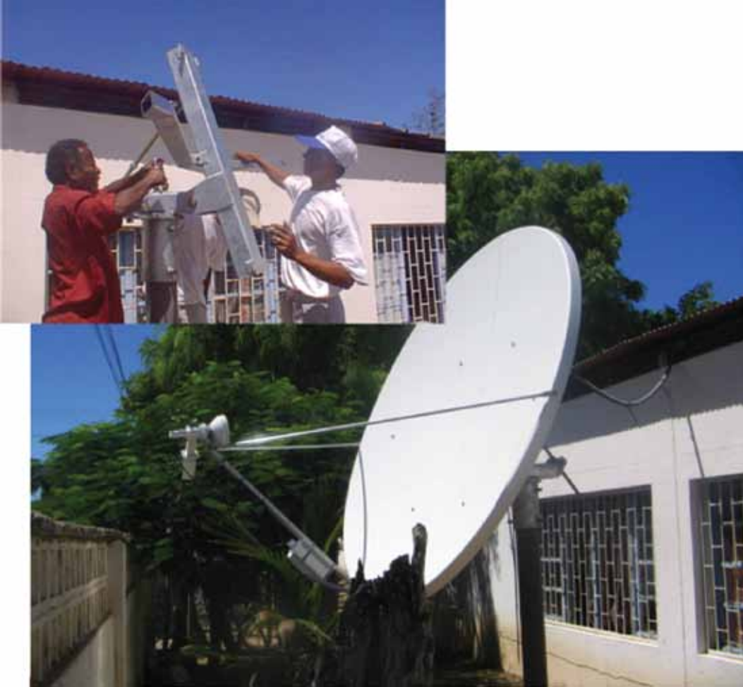
Figure 3. Installation of equipment for VSAT internet access at IHSM, Tulear, Madagascar.
