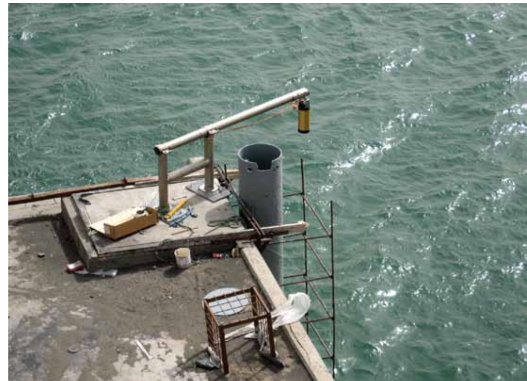
Figure 1. Tide gauge installation at Nouakchott port .
