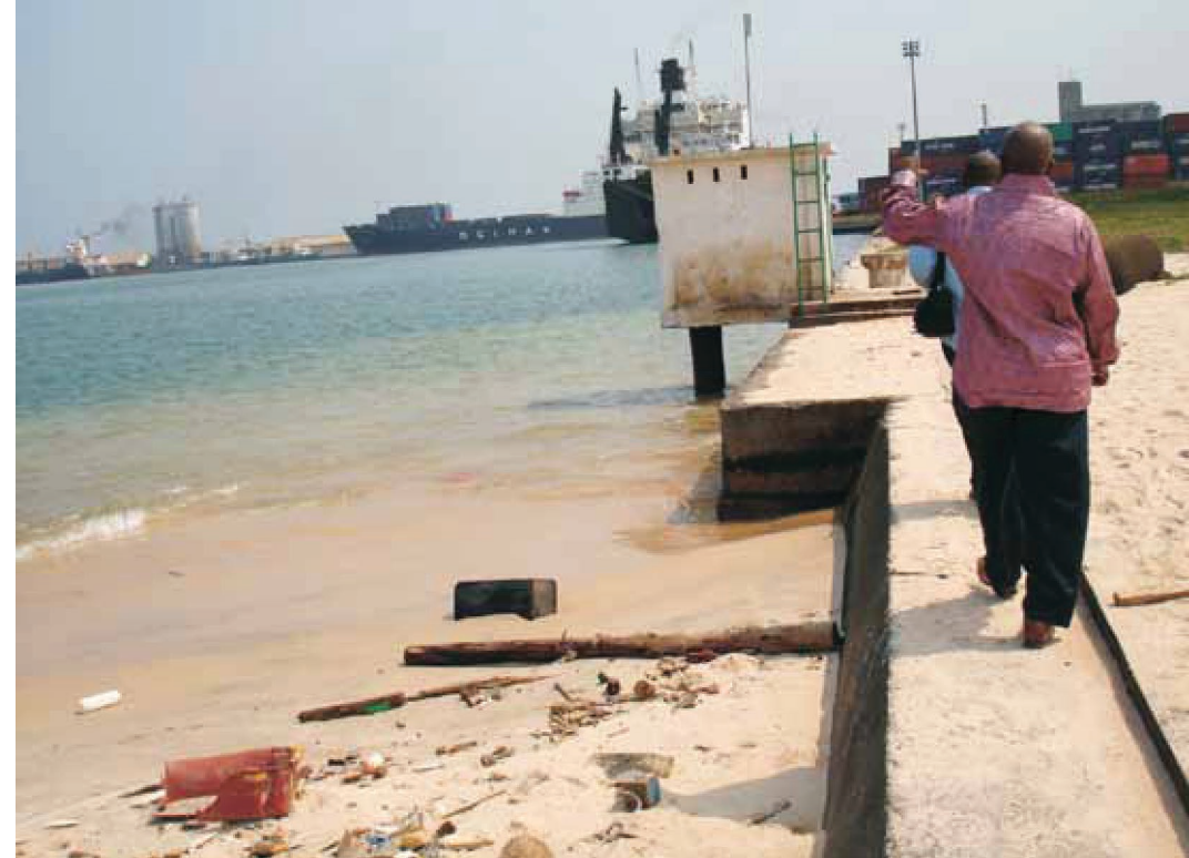
Figure 3. Example of erosion on the Congolese coast.
