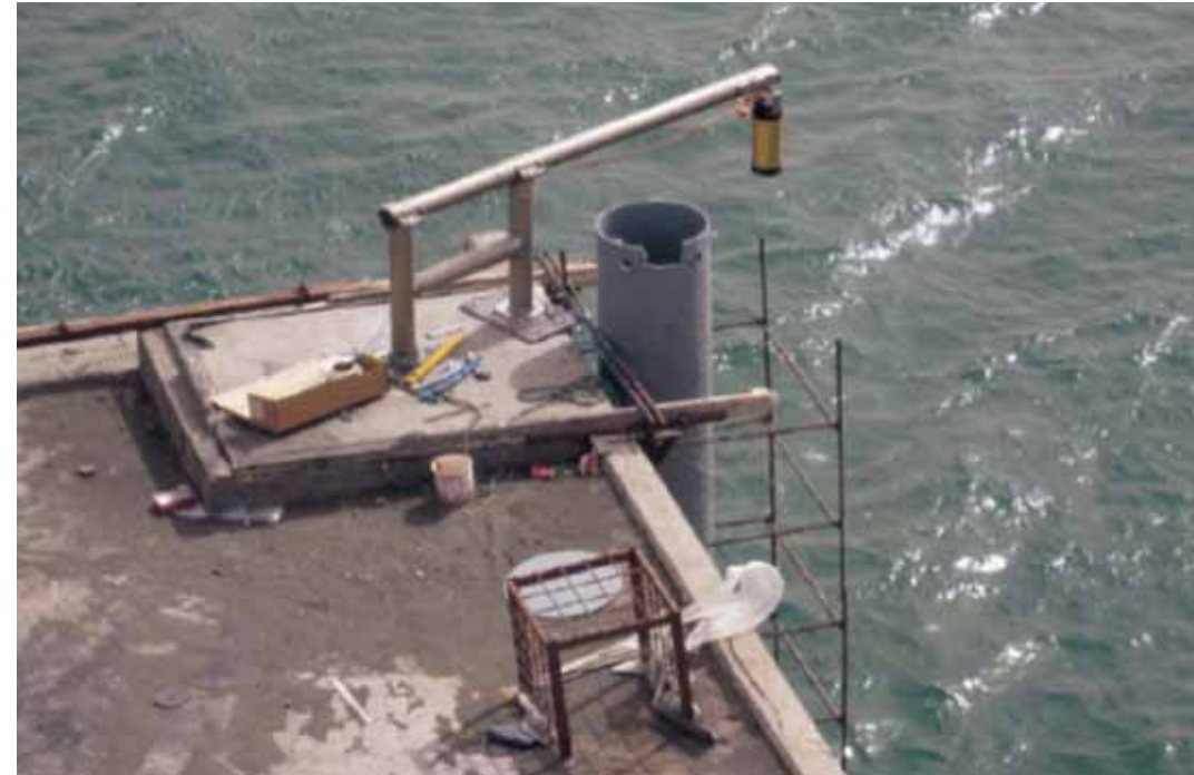
Figure 3. View of the radar sensor and aerials installation at Nouakchott station (Simon F., 2006).
