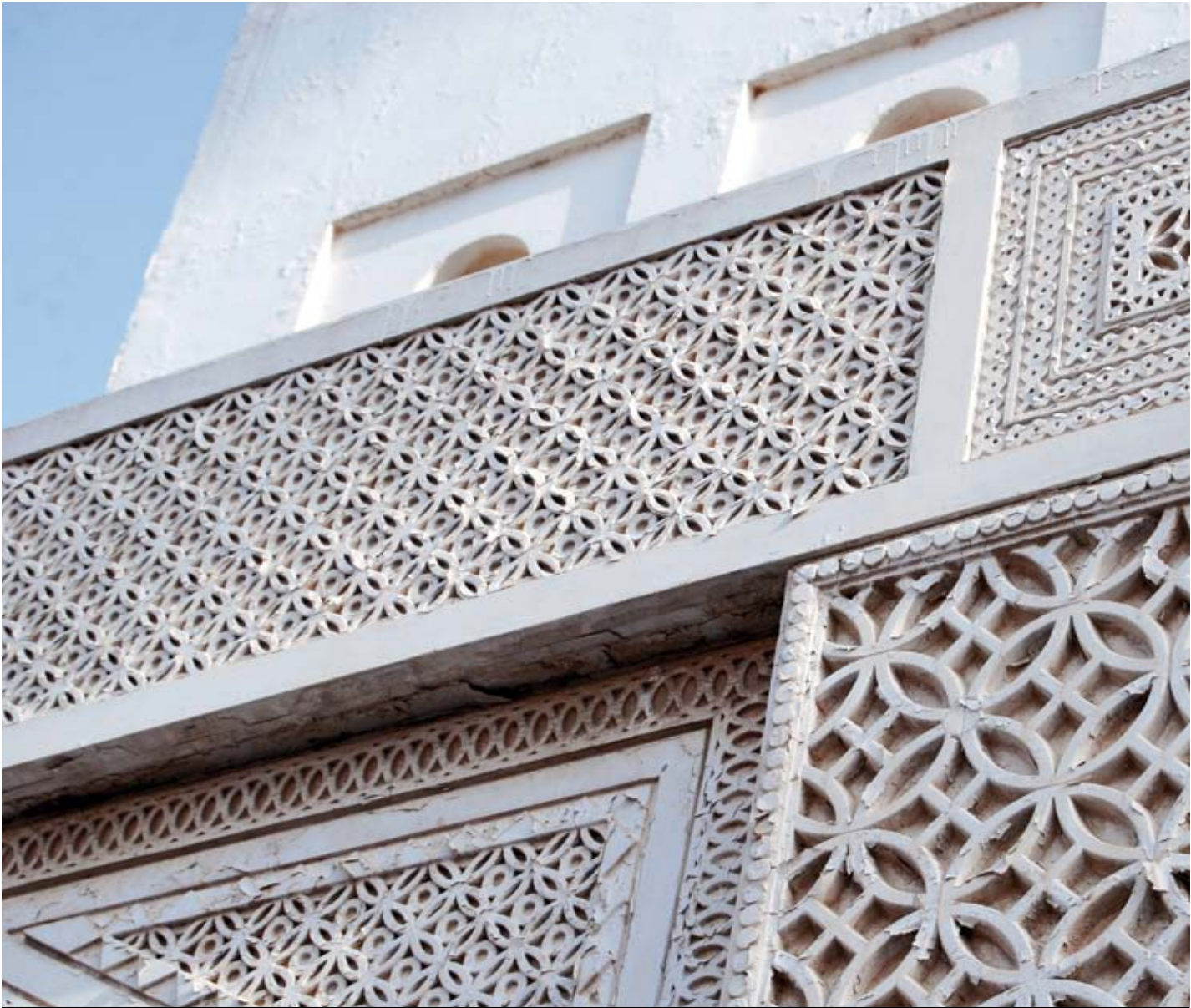
Detail of a 1970s carved gypsum ornament on outer façade of B01 - the North Gate.
