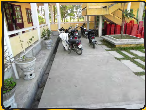
The picture above demonstrates how parked motorbikes and chairs block the entrance to the staircase. The playground has a wide drainage trench which is likely to cause accidents and injuries, especially when there is flooding and the ground is covered by water and people cannot see where they step.
