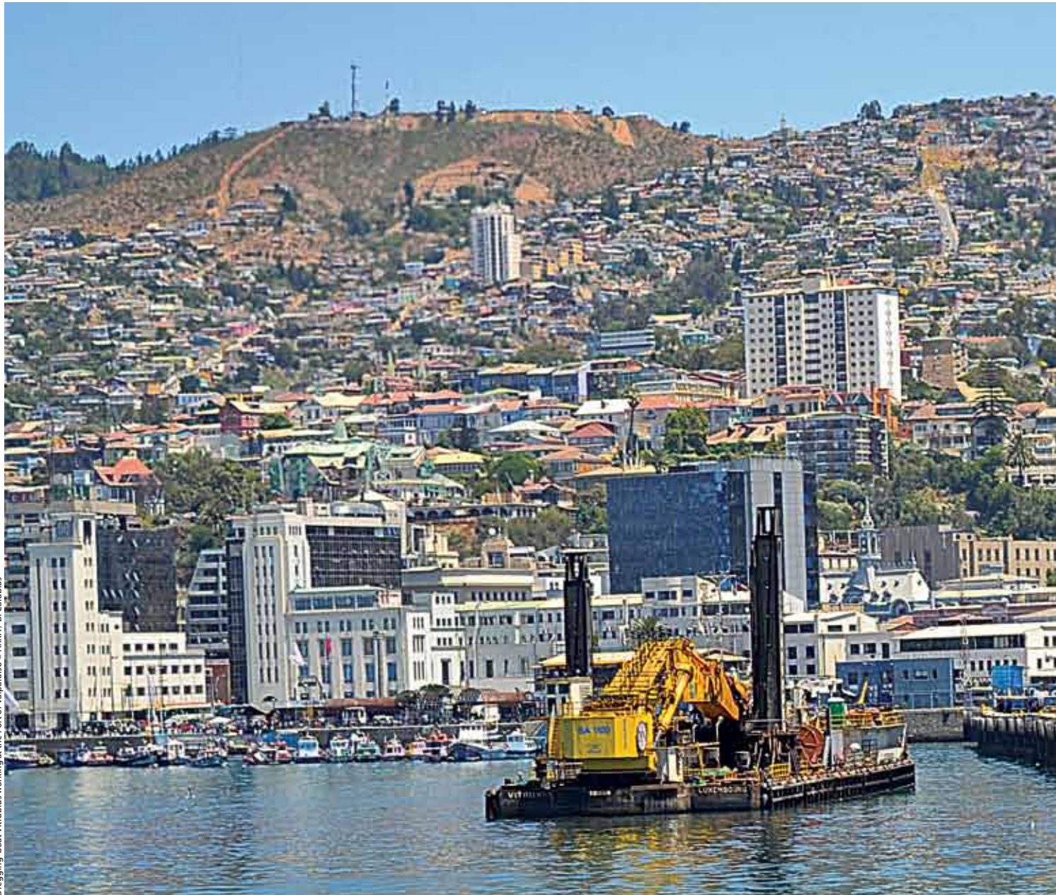
Dredging boat Vitruvius working at the Port of Valparaíso © ARKA / D. Carabias
